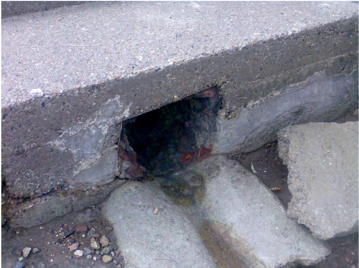
Figure XIII.3 Unidentified pipeline discharge at Wells Quay.
