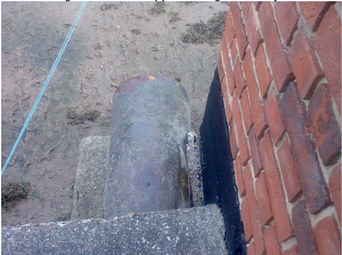
Figure XIII.4 Unidentified pipeline discharge at Wells Quay.
