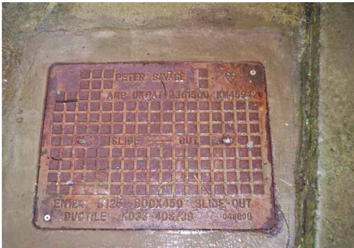
Figure XII.7 Man-hole cover for sewer at Kingswear.
