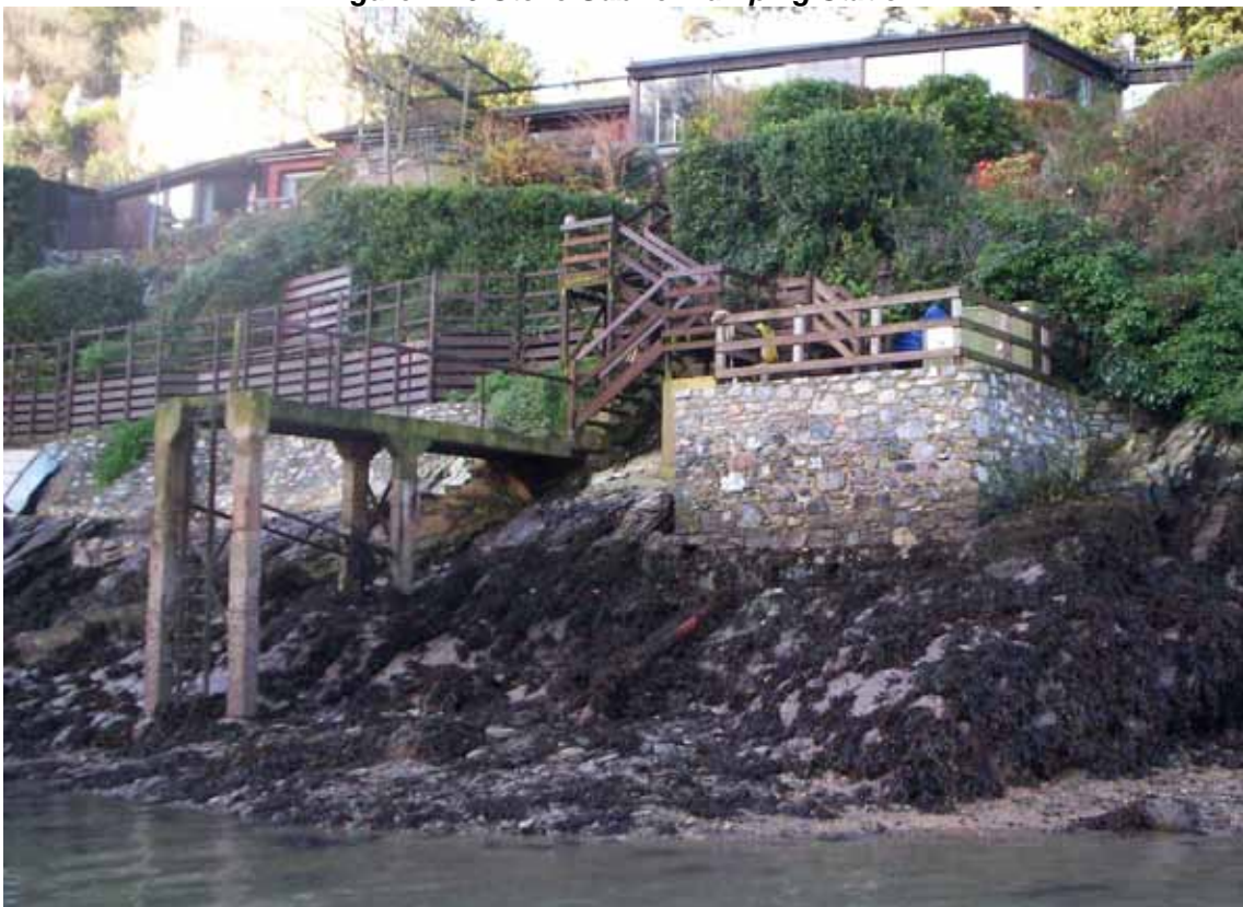
Figure XII.10 Unidentified piped discharge at Warfleet Creek.
