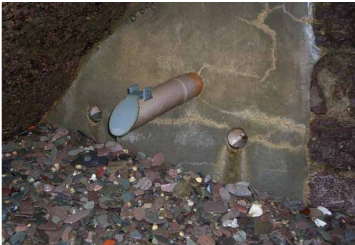
Figure XII.6 Unidentified piped discharge at Kingswear (SX8826550878).
