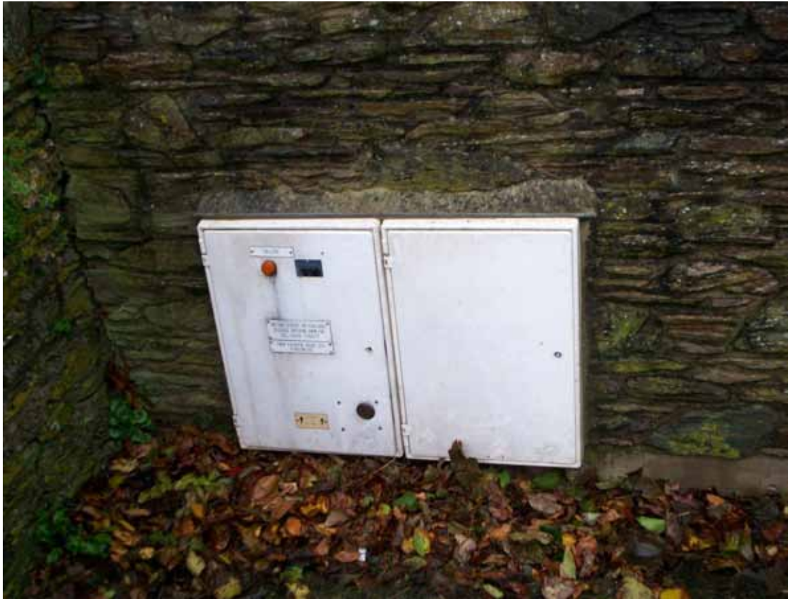
Figure XII.3 Yarrow Bank Pumping Station.
