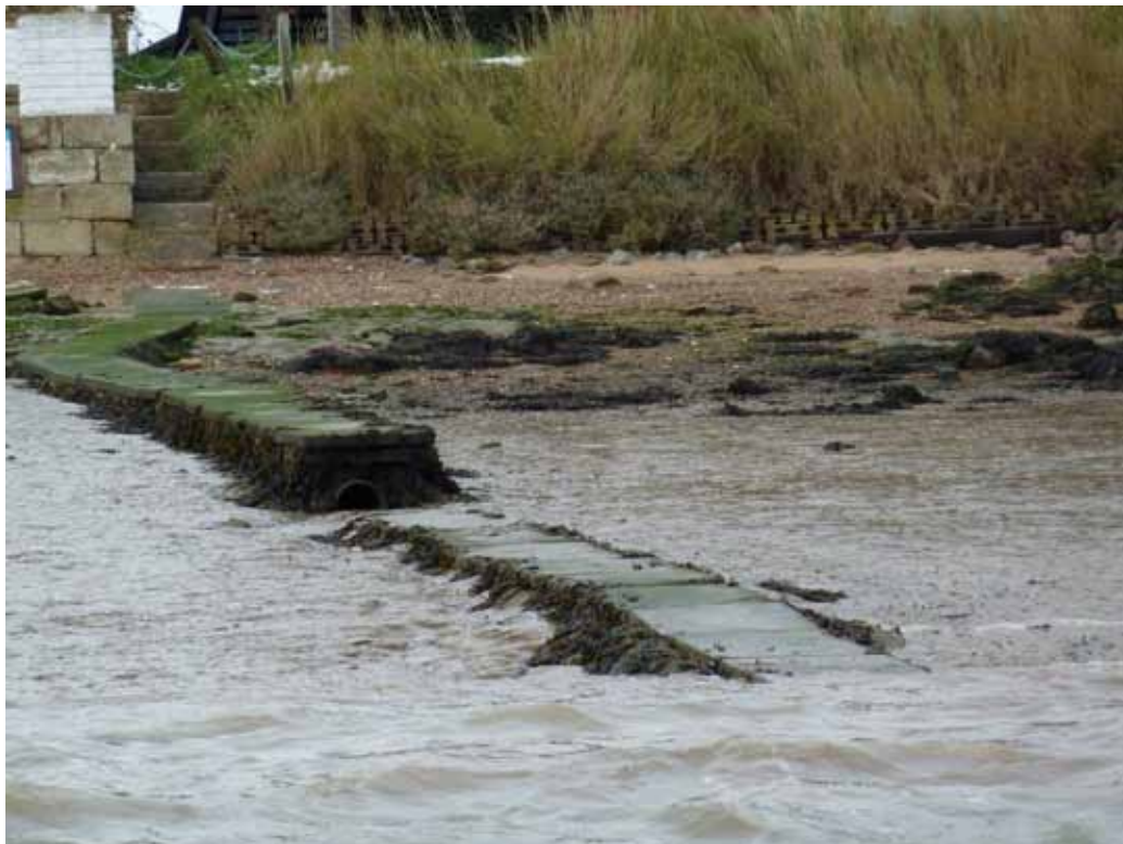
Figure XIV.6 – Surface outfall pipe at Waldringfield
