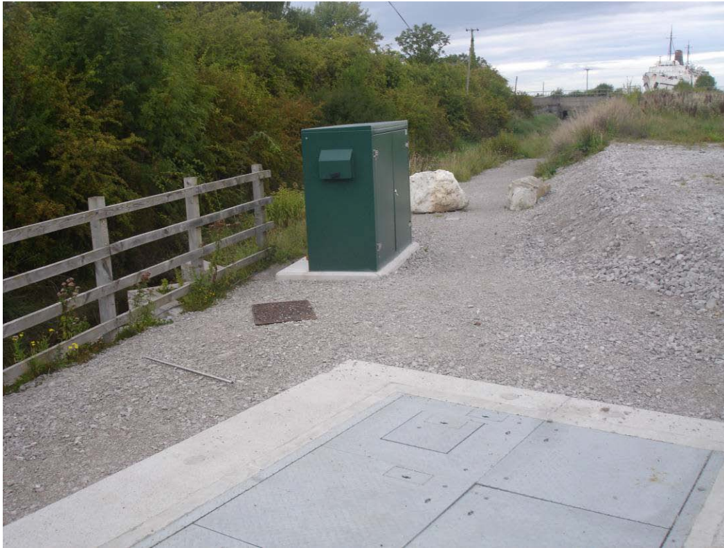
Figure XII.9 – Sewage pumping station adjacent to stream
