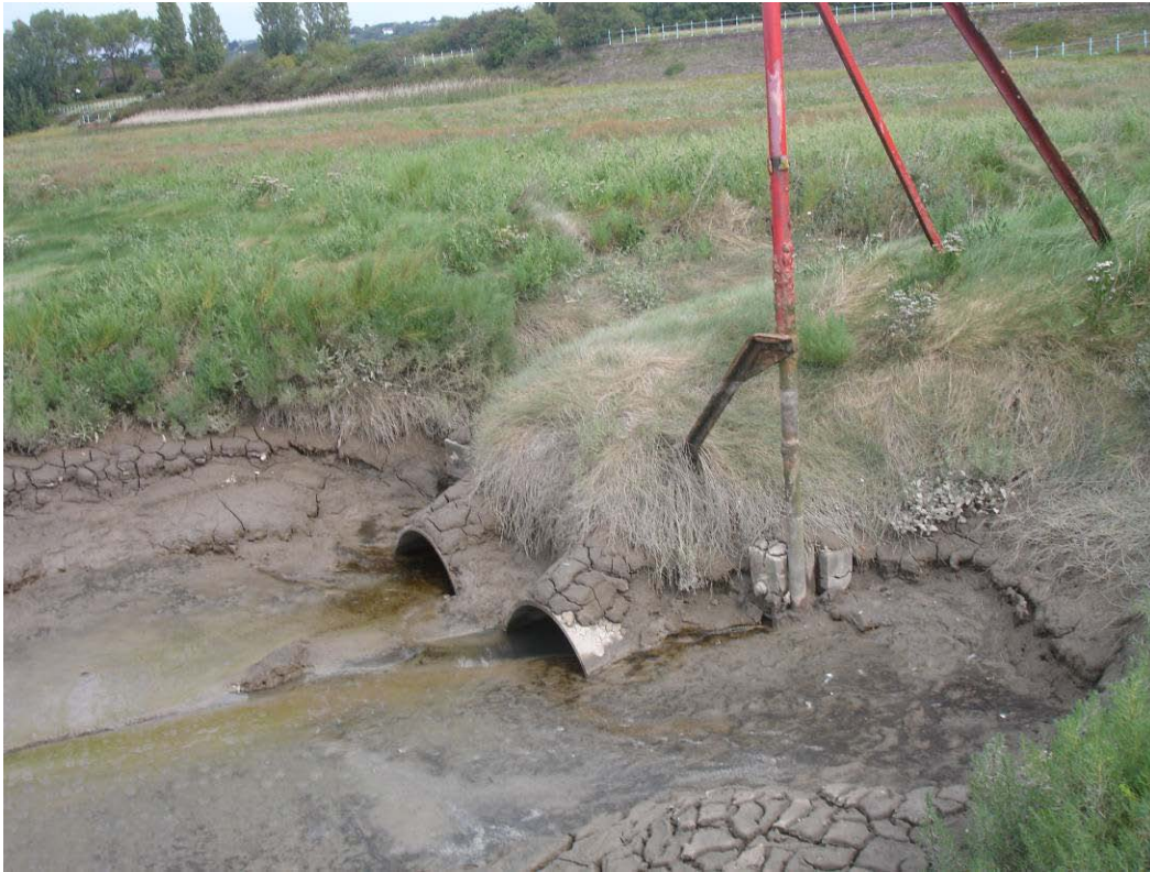
Figure XII.5 – Heswall storm tank CSO outfalls
