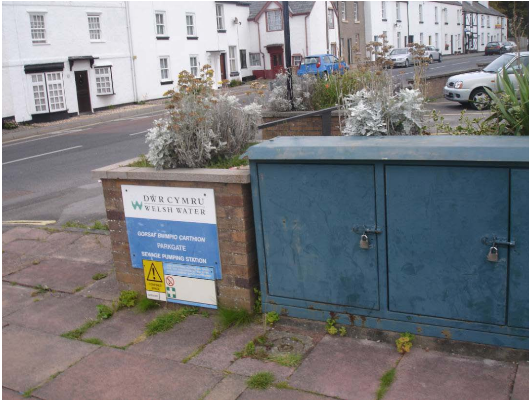
Figure XII.3 –Parkgate SPS enclosure
