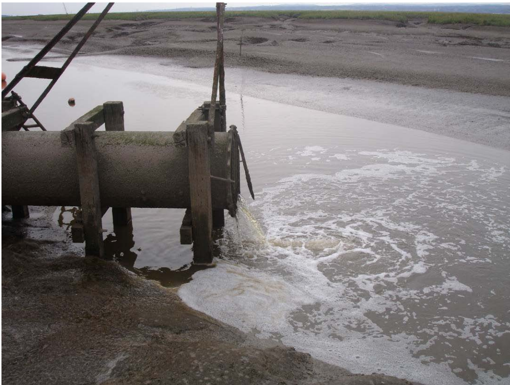
Figure XII.6 – Heswall STW main outfall to creek
