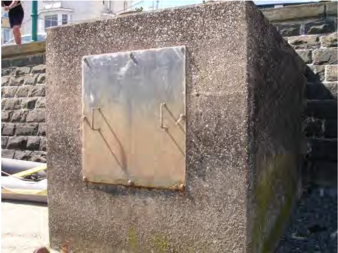
Figure XIII.5 Aberdify Wharf emergency overflow.
