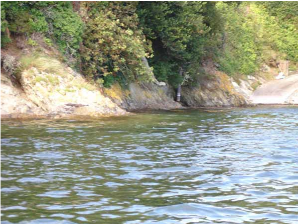
Figure XIII.13 Piped discharge at St. Just.
