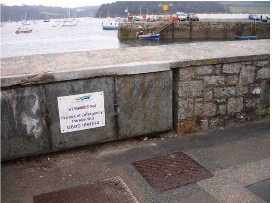
Figure XIII.14 St. Mawes PS No1 control box.
