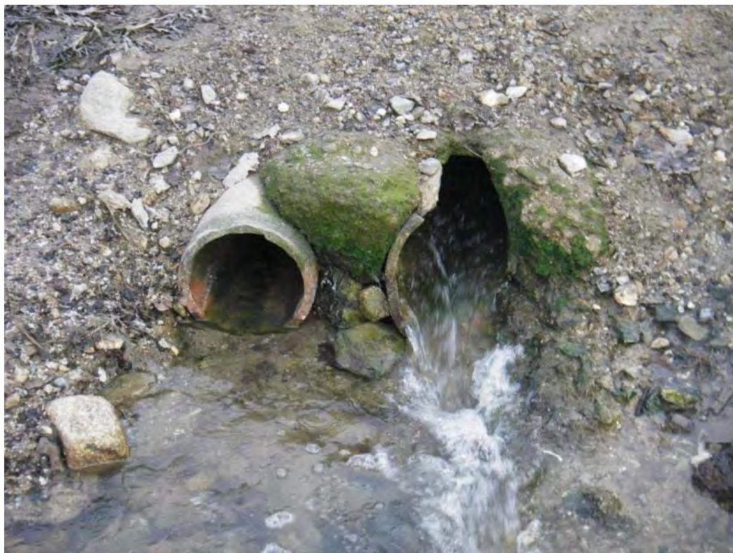
Figure 78. Pipes on Cowlands Creek at Coombe
