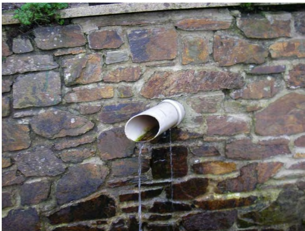
Figure 75. Dripping pipe at King Harry Ferry slipway
