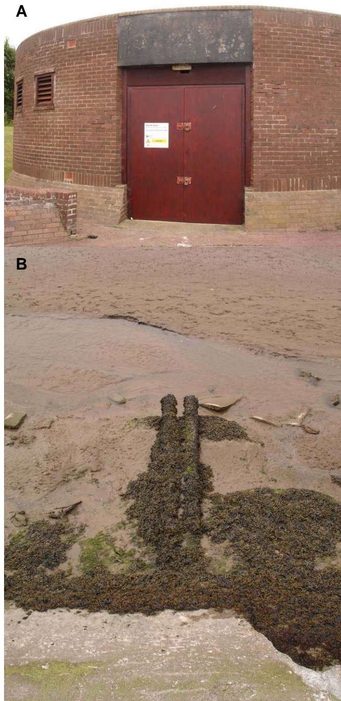
Figure XIII.3 Observed discharges. A – Meols WWTW pumping station. B – Cast iron pipes from sea wall at Meols.
