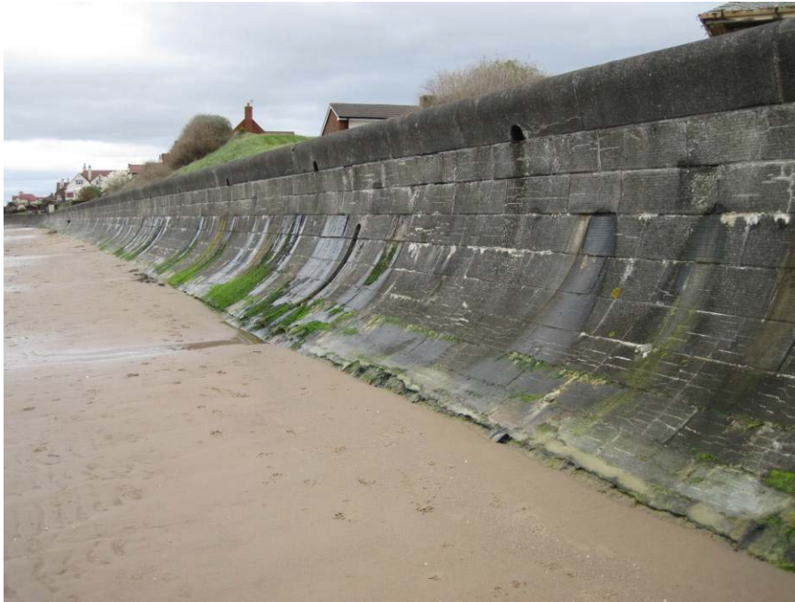
Figure I.1: Ground water seeping through sea defences along the north Wirral coast.
