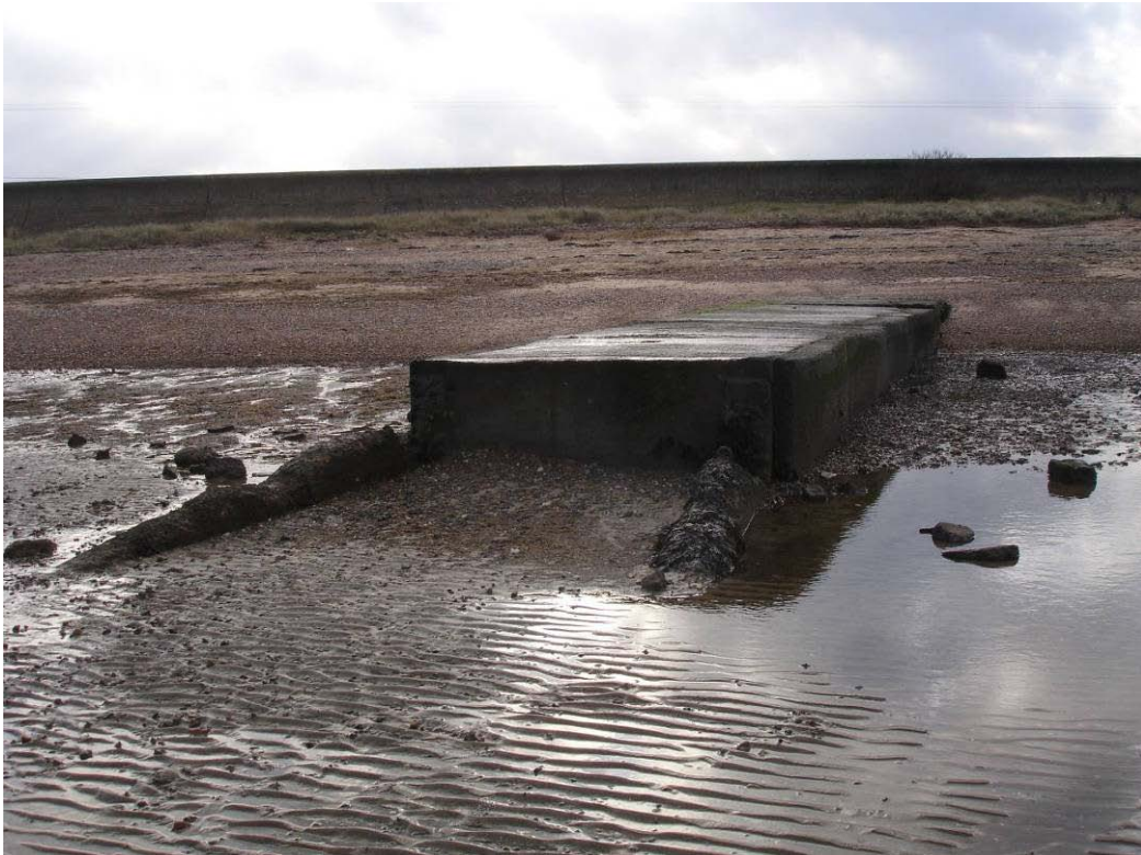
Figure XIII.22 Blocked surface water outfall
