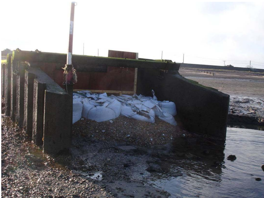
Figure XIII.21 Blocked surface water outfall
