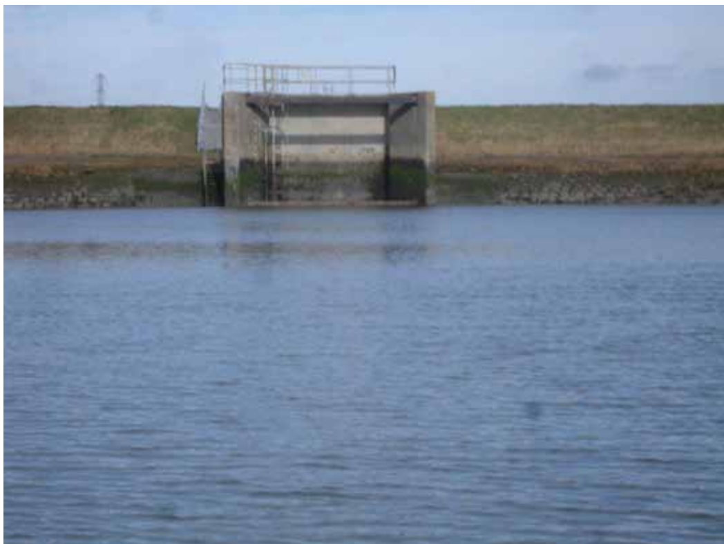
Figure XIV.4 Sluice at head of Clementsgreen Creek
