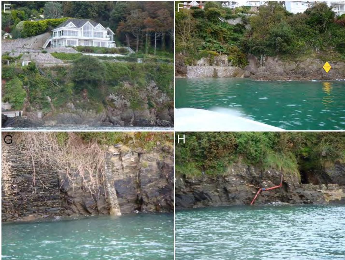
Figure A3-2 Unidentified piped discharges inspected during the shoreline survey on 1 October 2008.
