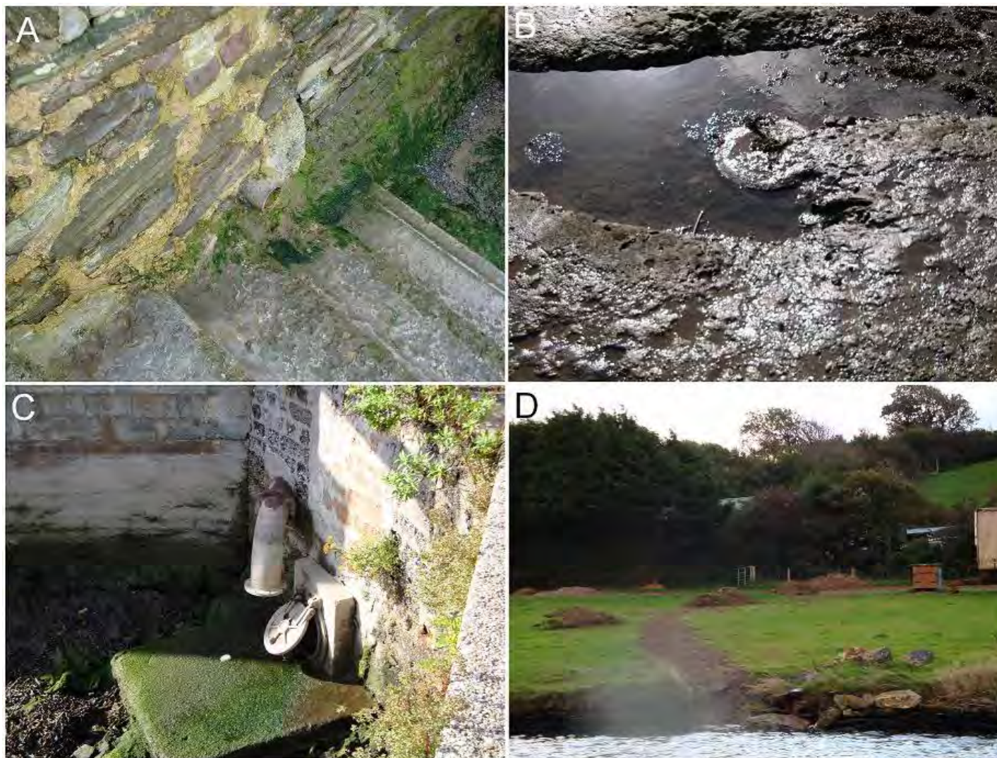
Figure A3-1 Unidentified piped discharges inspected during the shoreline survey on 1 October 2008.
