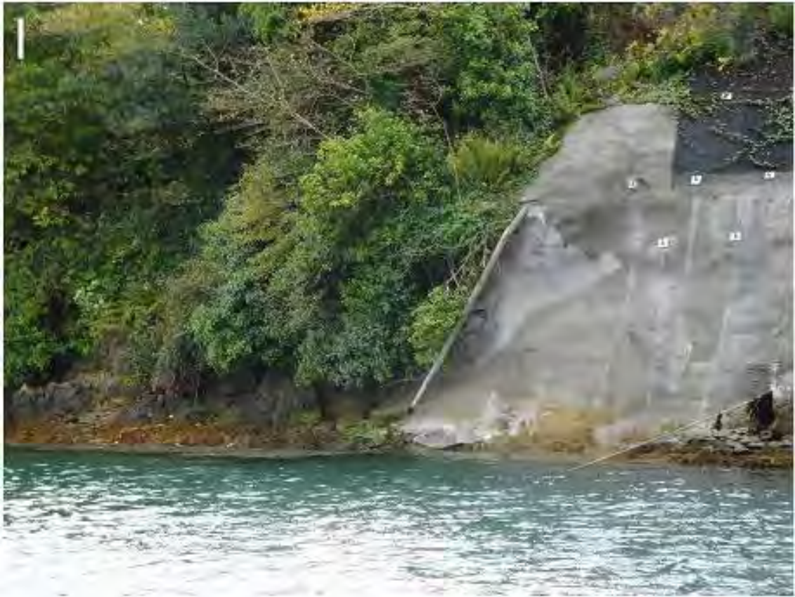
Figure A3-3 Unidentified piped discharge inspected during the shoreline survey on 1 October 2008.
