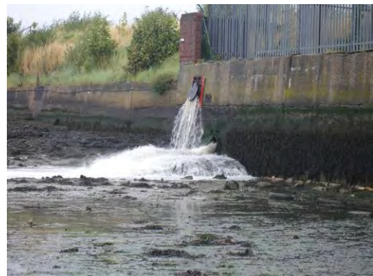
12: Woolston STW storm overflow
