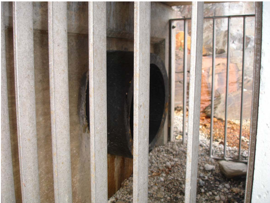
Figure XIII.11 Unidentified pipe at Duporth Beach (03448/51092).
