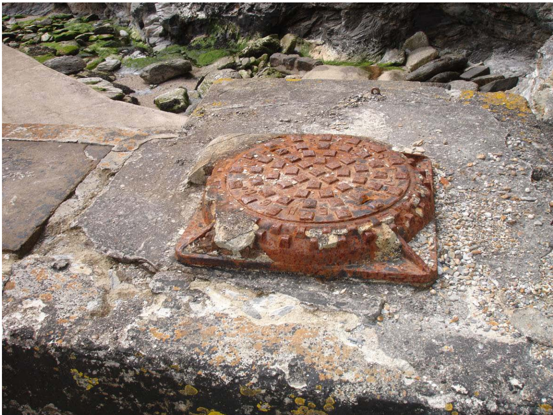
Figure XIII.5 Manhole cover at Charlestown Harbour PS CSO/EO.
