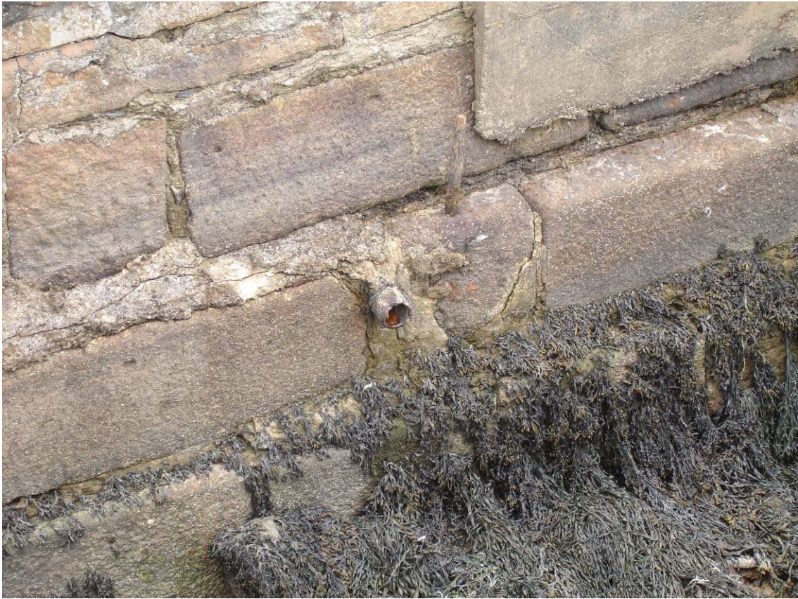
Figure XIII.10 Unidentified piped discharge at Par Docks (03917/51549).
