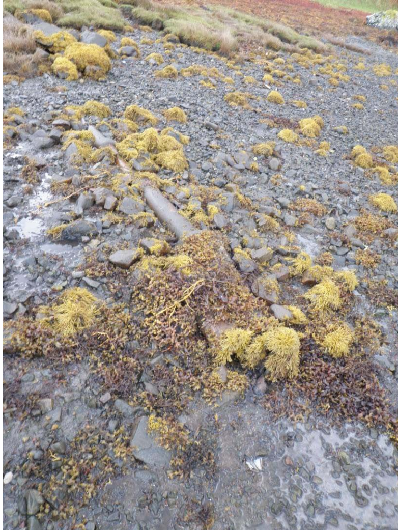
Figure 15 Discharge pipe on shore at Camas an t-Salainn
