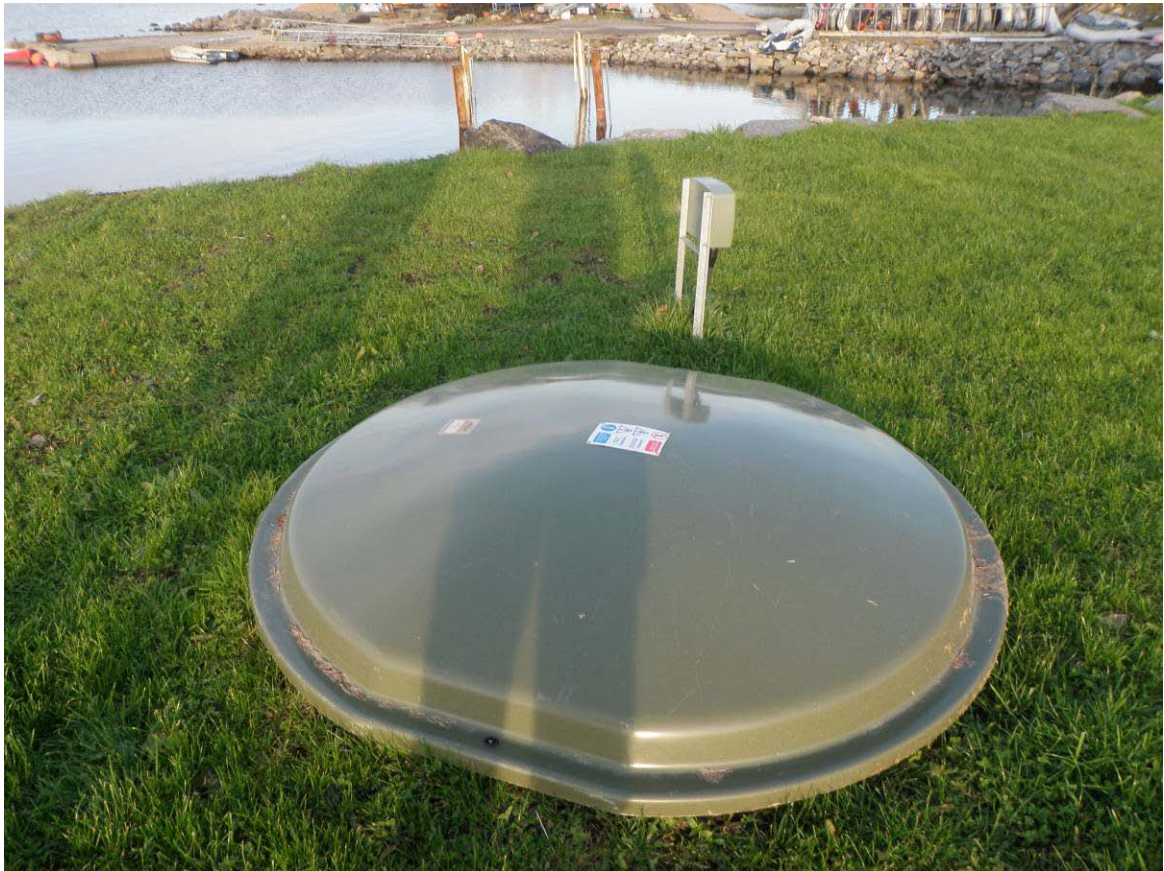
Figure 21 Septic tank at boatyard
