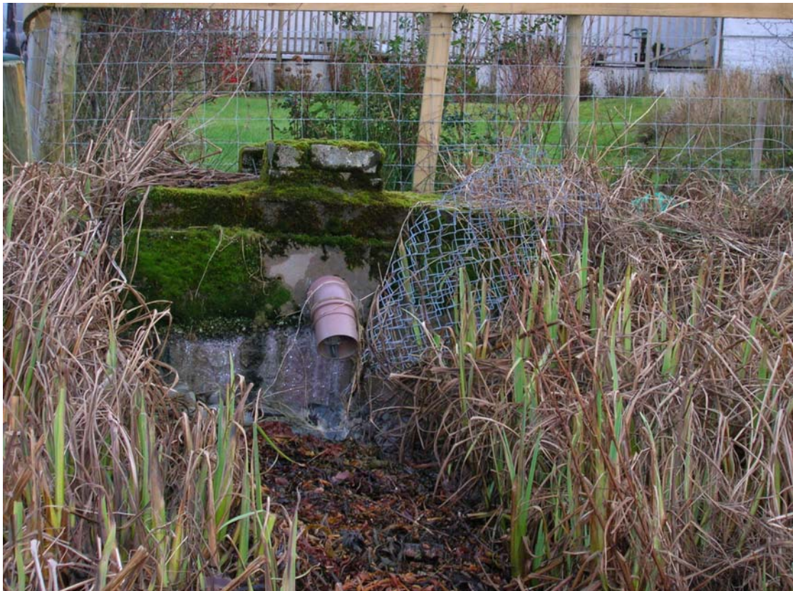
Figure 9. Dripping overflow from Morar septic tank
