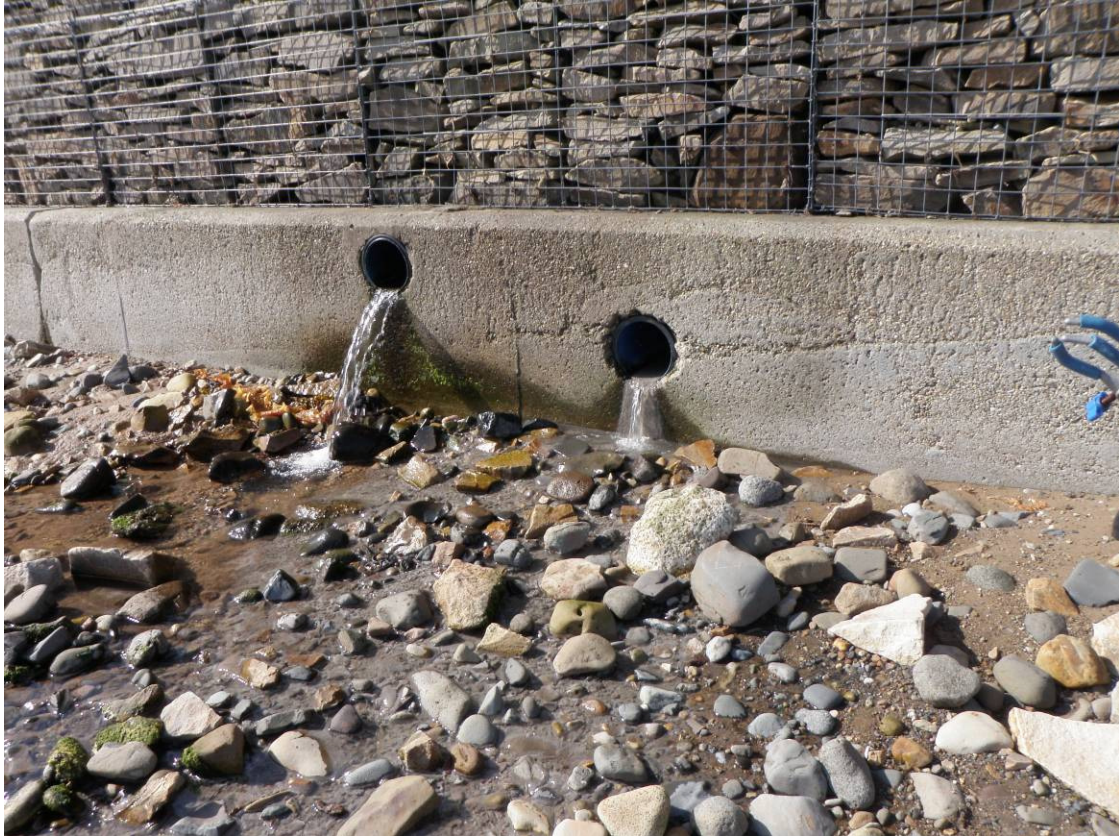
Figure 23. Two pipe below Whiting Bay PS2, water samples 42 & 43
