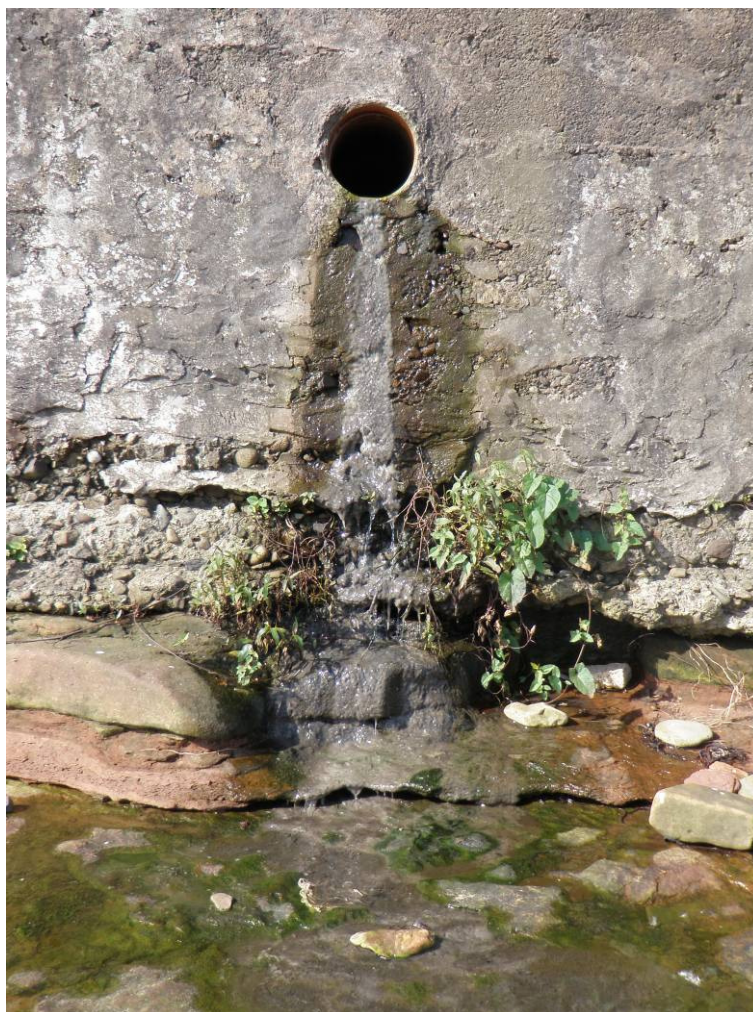
Figure 22. Pipe coming out of wall, sewage fungus, water sample 39
