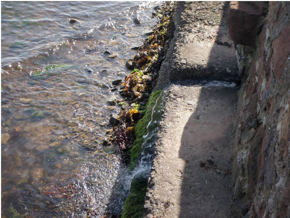
Figure 24. Concrete pipe flowing into sea, very strong smell of sewage, water sample 45
