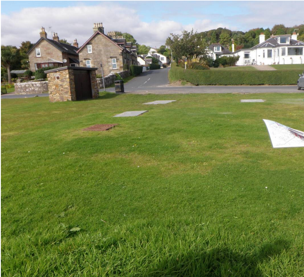
Figure 14. Lamlash PS3, electrical unit and 4 inspection covers in the ground
