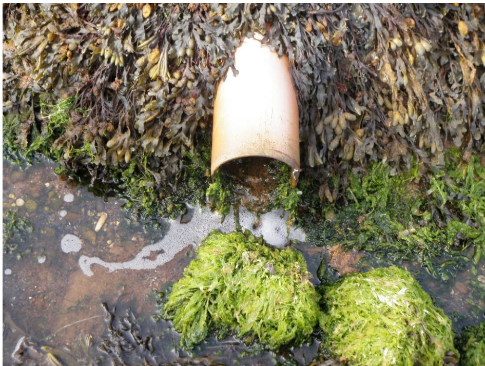
Figure 16. Pipe encased in concrete, flowing under water, water sample 24
