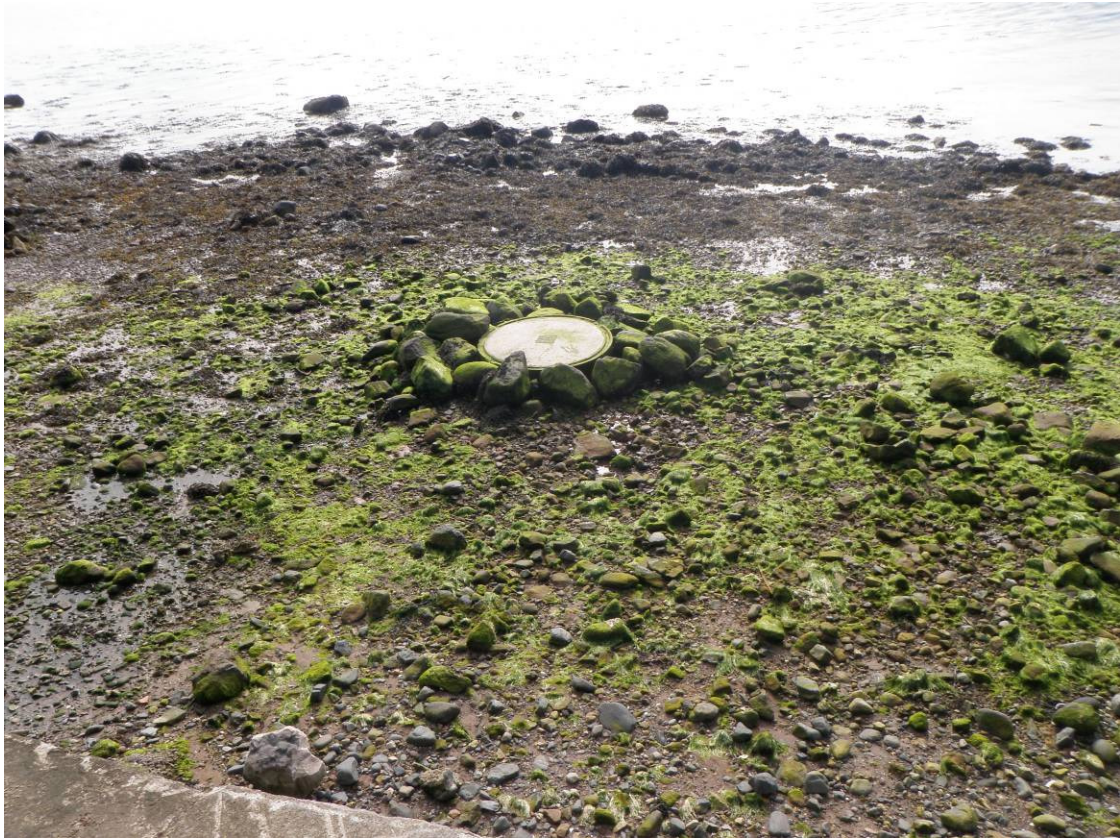
Figure 12. Inspection cover covered in algae
