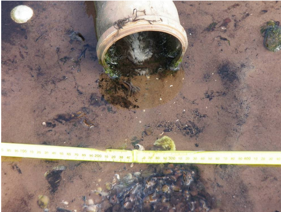
Figure 10. Pipe with sewage fungus inside, flow too small to sample
