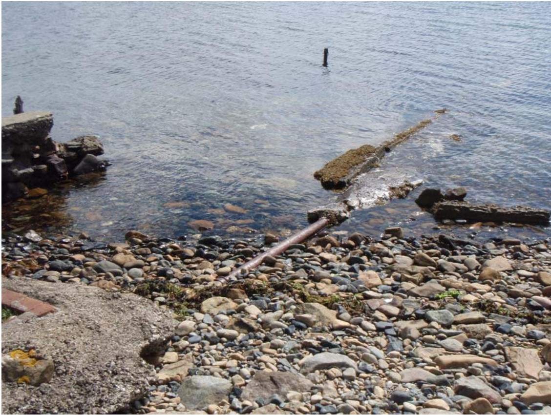
Figure 8. Private sewer outfall
