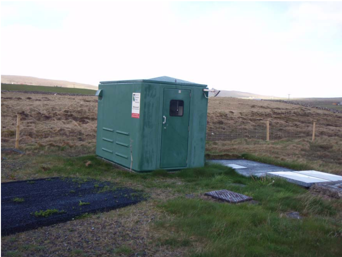
Figure 13. Scottish Water pumping station
