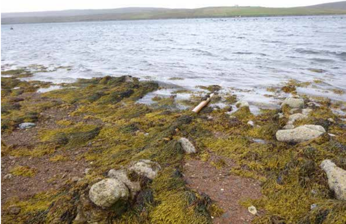
Figure 10 – Discharge pipe to sea associated with the septic tank of the disused North Isles Motel.
