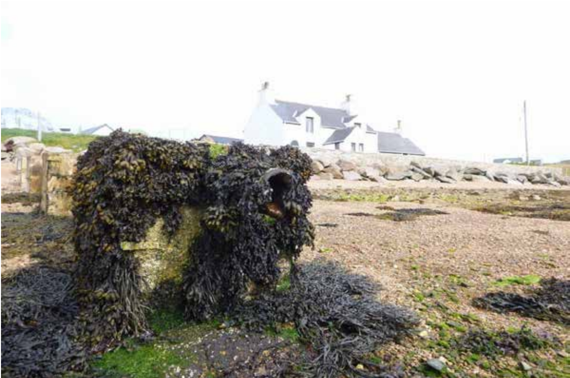
Figure 9 – The outfall associated with the septic tank illustrated in Figure 8.
