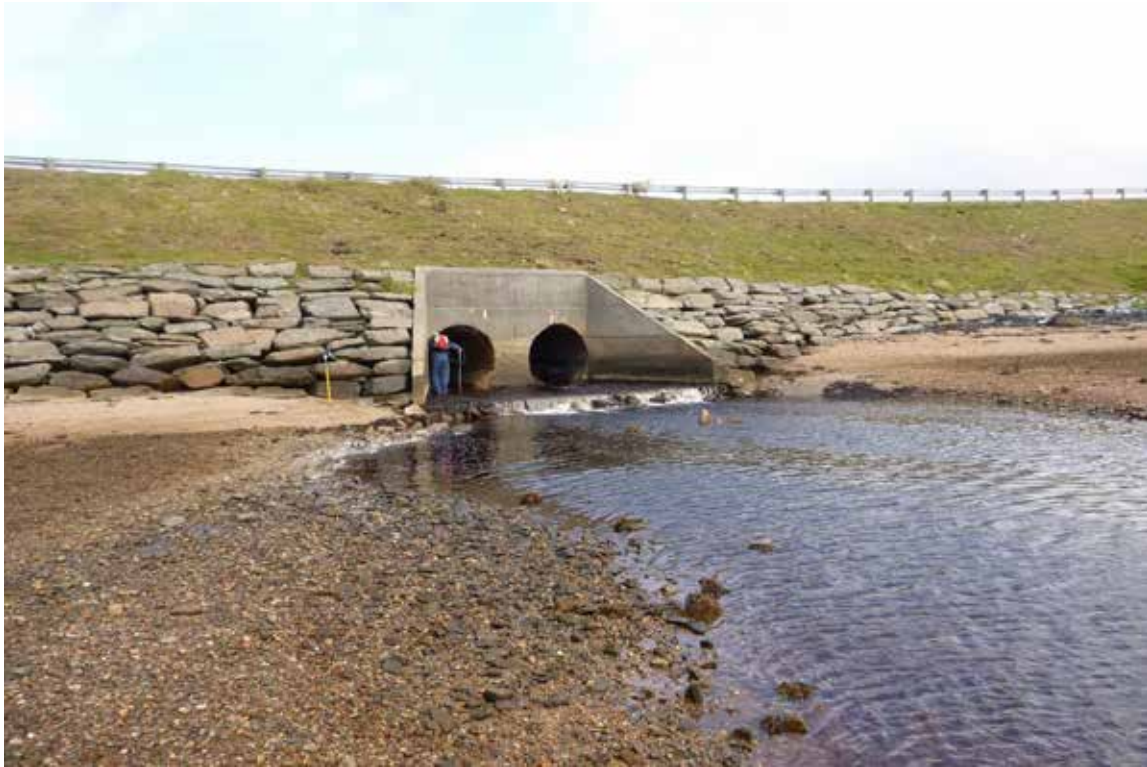
Figure 14 – Culvert for the Burn of Gossawater under the A968 road at the head of Basta Voe.
