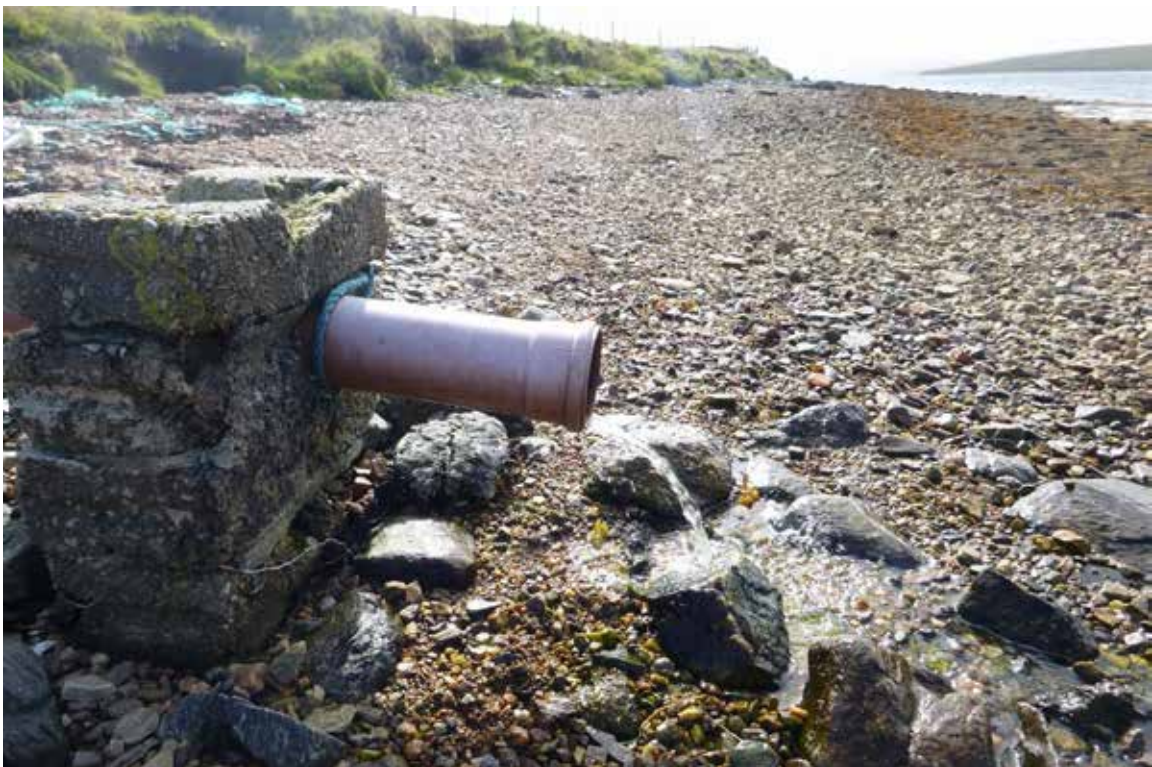
Figure 11 – Pipe with clear discharge. No source identified, potentially field drainage.
