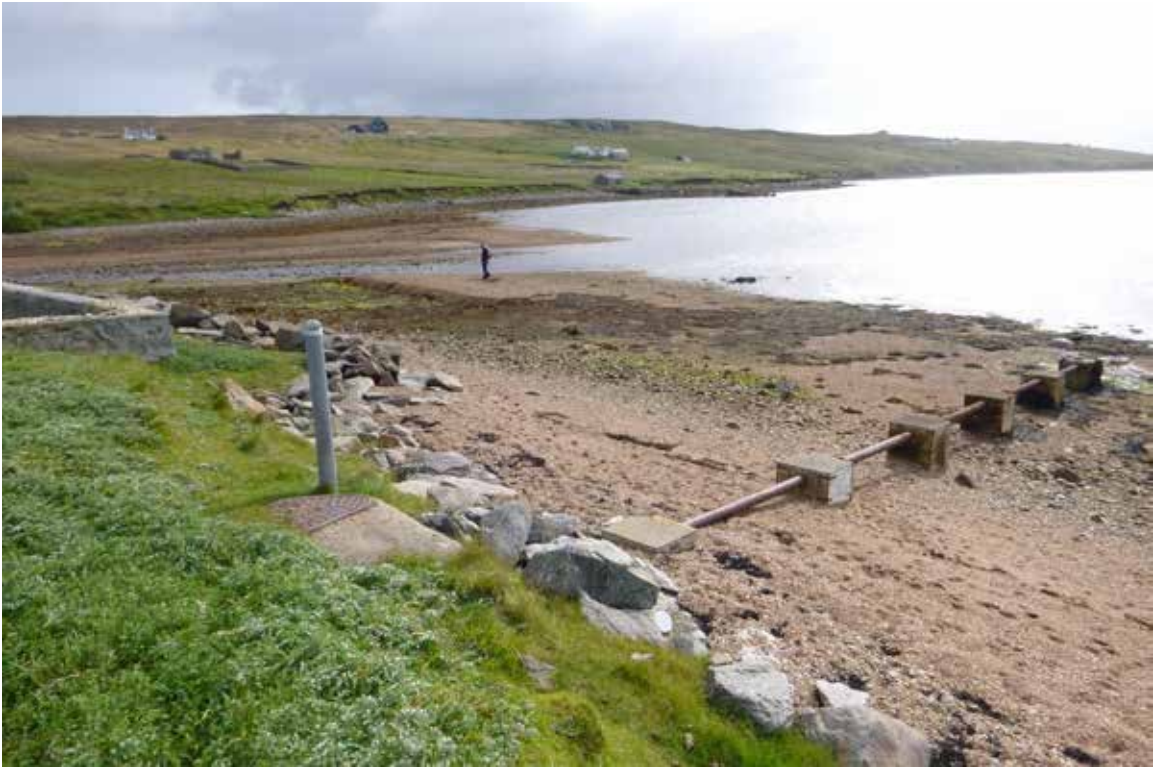
Figure 8 – Concrete septic tank and outfall associated with property close to shore. Sandwater Burn beyond.
