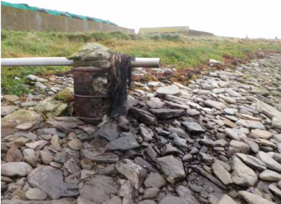
Figure 9. Silage effluent pipe at Elsness
