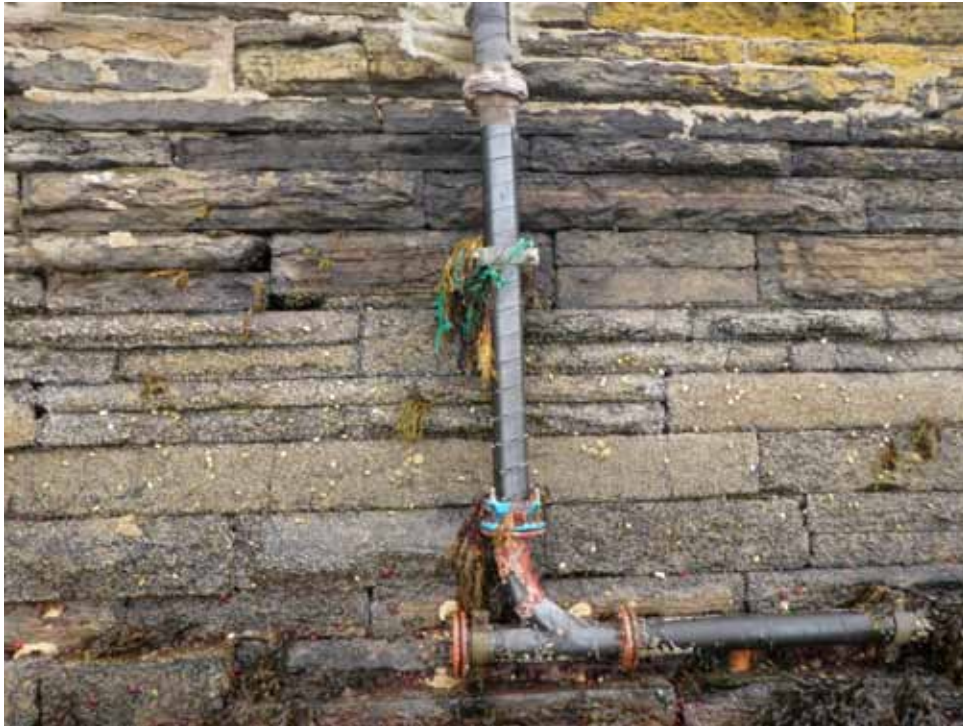
Figure 7. Pipe behind facilities at Kettletoft pier
