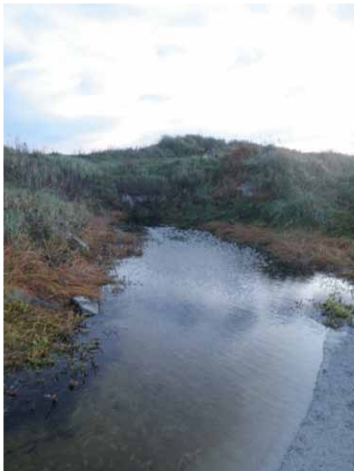
Figure 10. Water puddled next to sand berm
