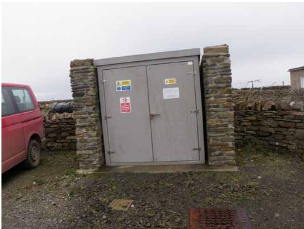
Figure 4. Scottish Water ST and pumping station
