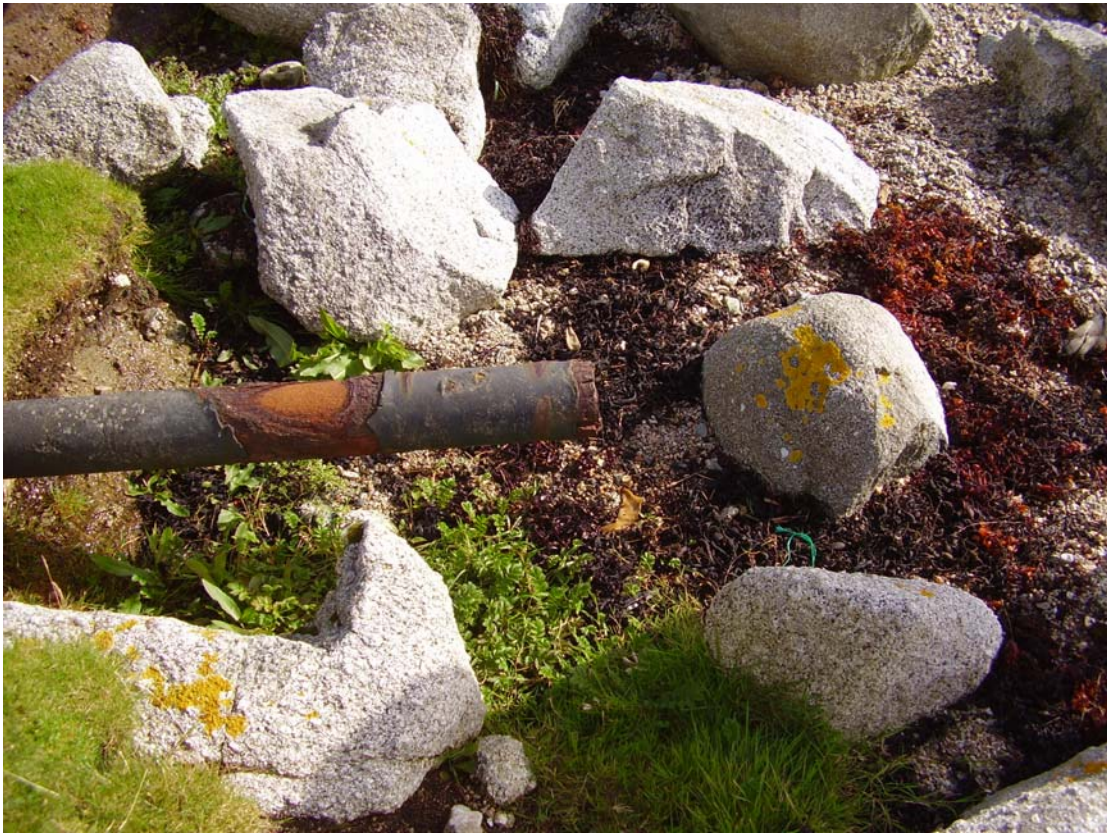
Figure 14. Busta050912. Discharge pipe.
