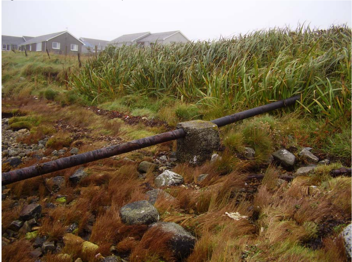
Figure 22. Busta060909. Pipe across shoreline.
