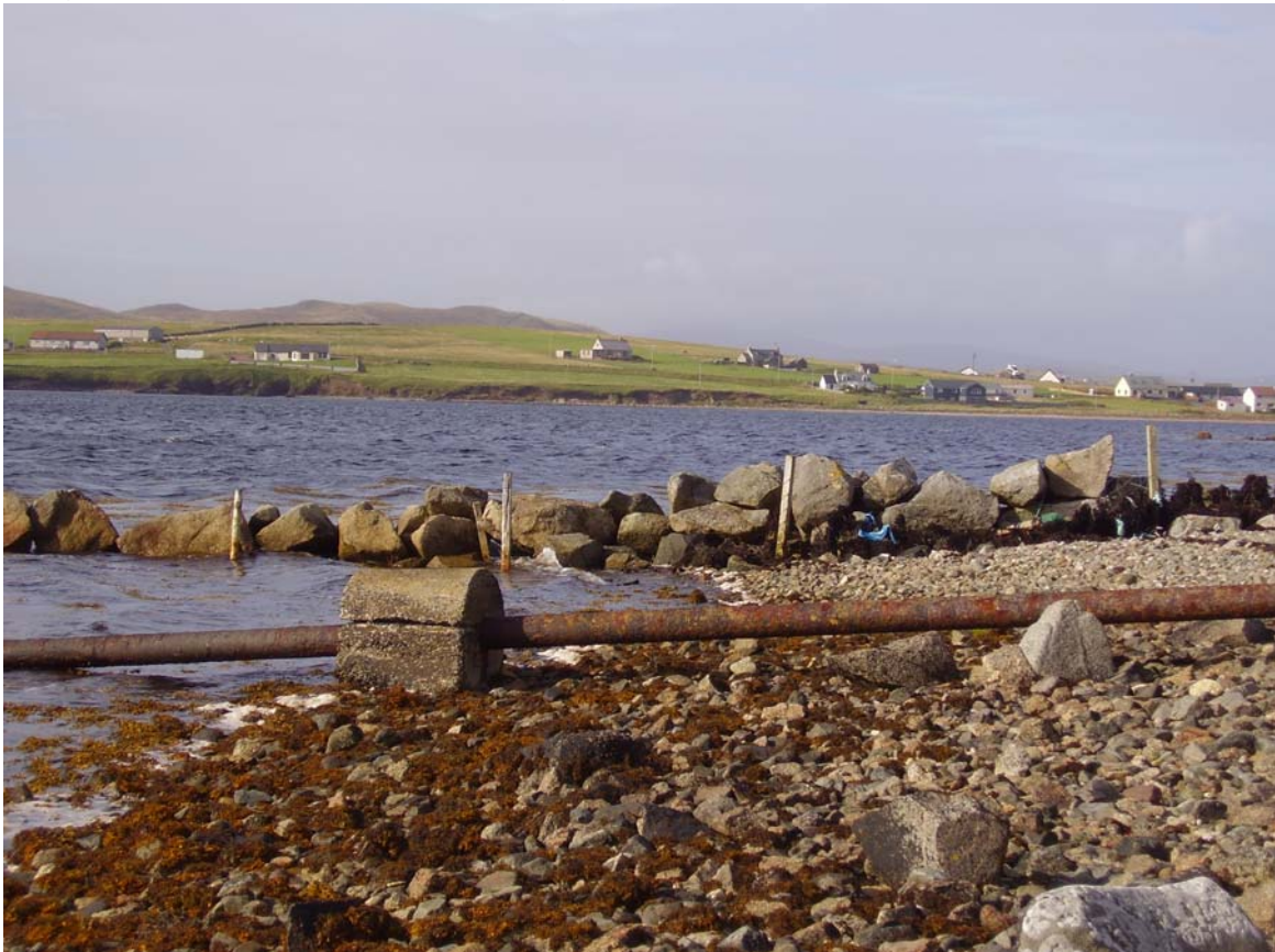
Figure 15. Busta050913. Discharge pipe.
