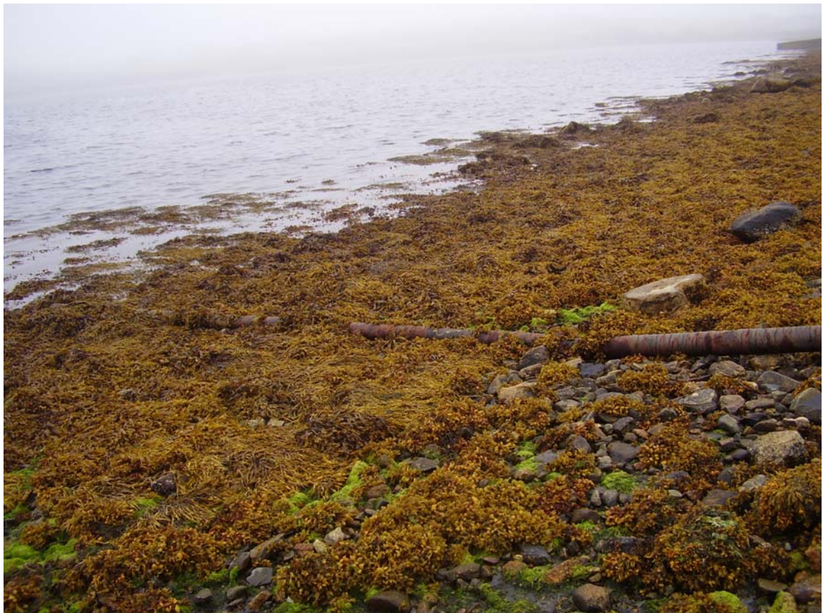
Figure 23. Busta060910. Broken pipe on shore.
