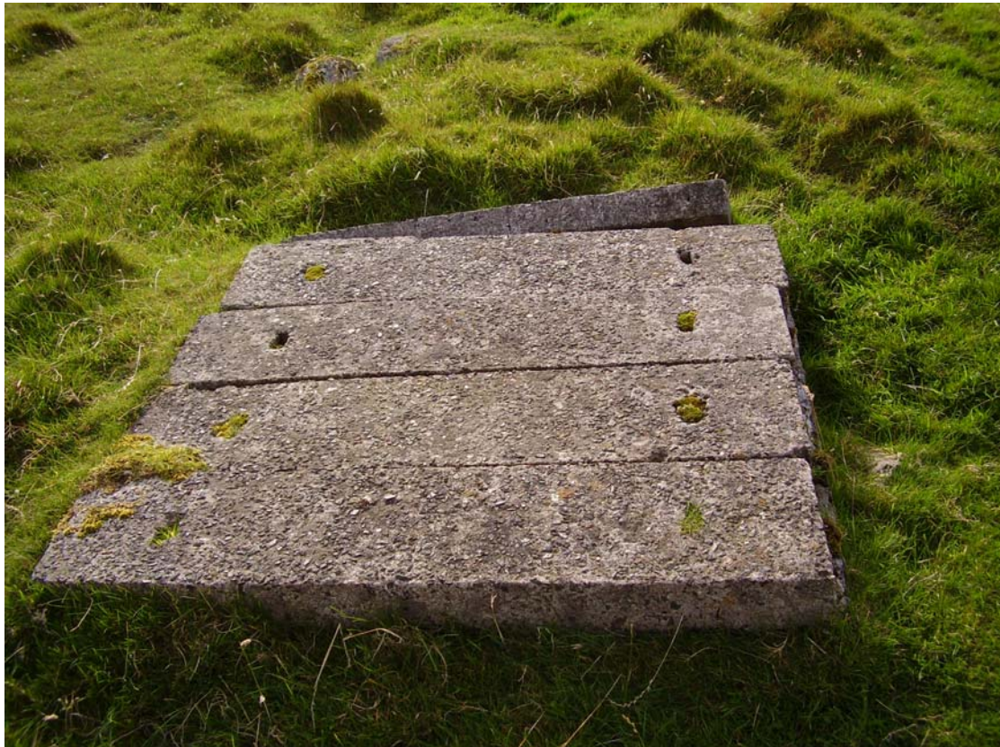
Figure 16. Busta050911. Concrete septic tank cover.
