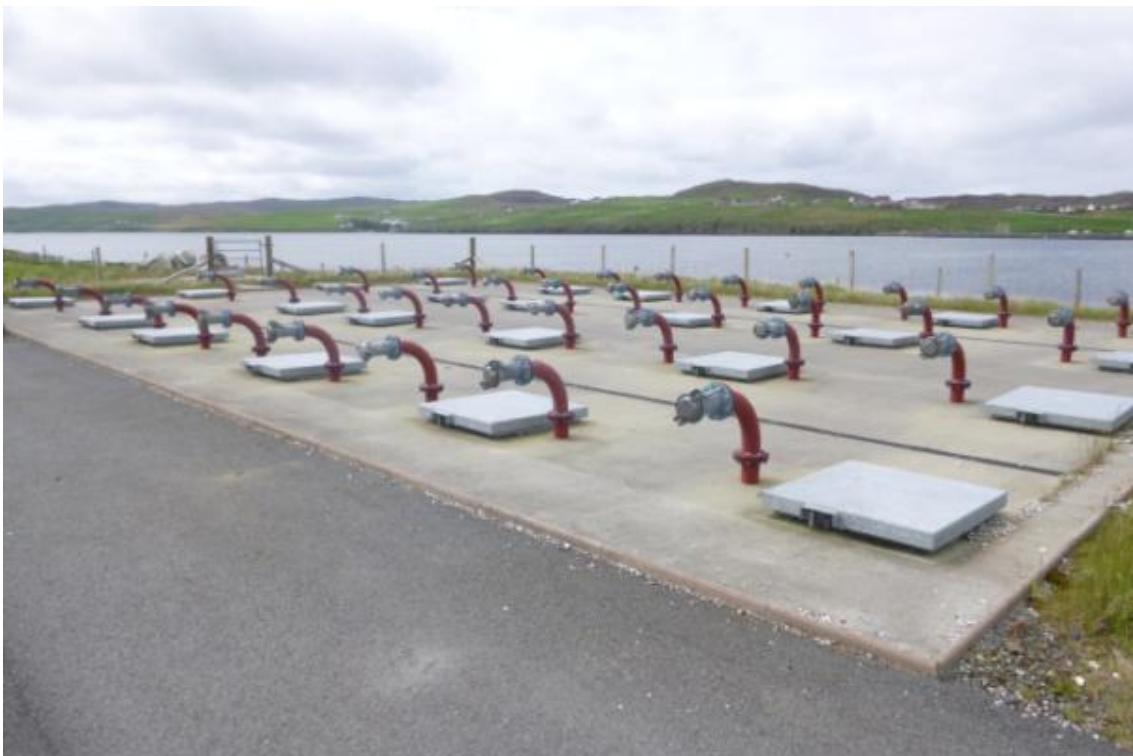
Figure 9 – Brae community septic tank.
