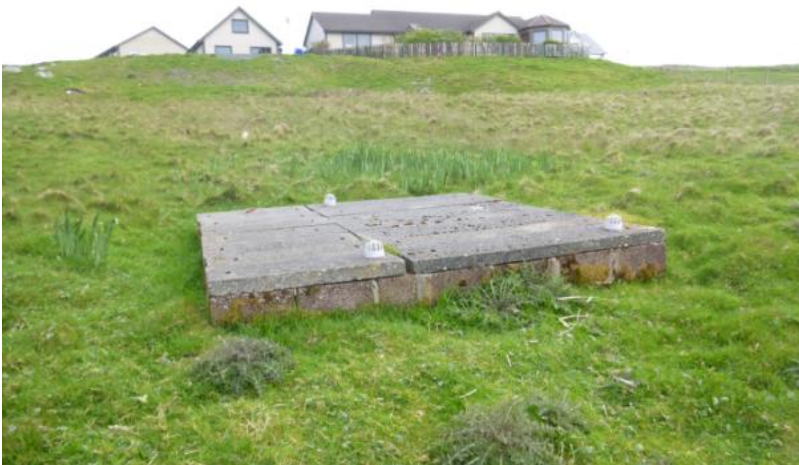
Figure 13 – Septic tank associated with houses at Sparl.
