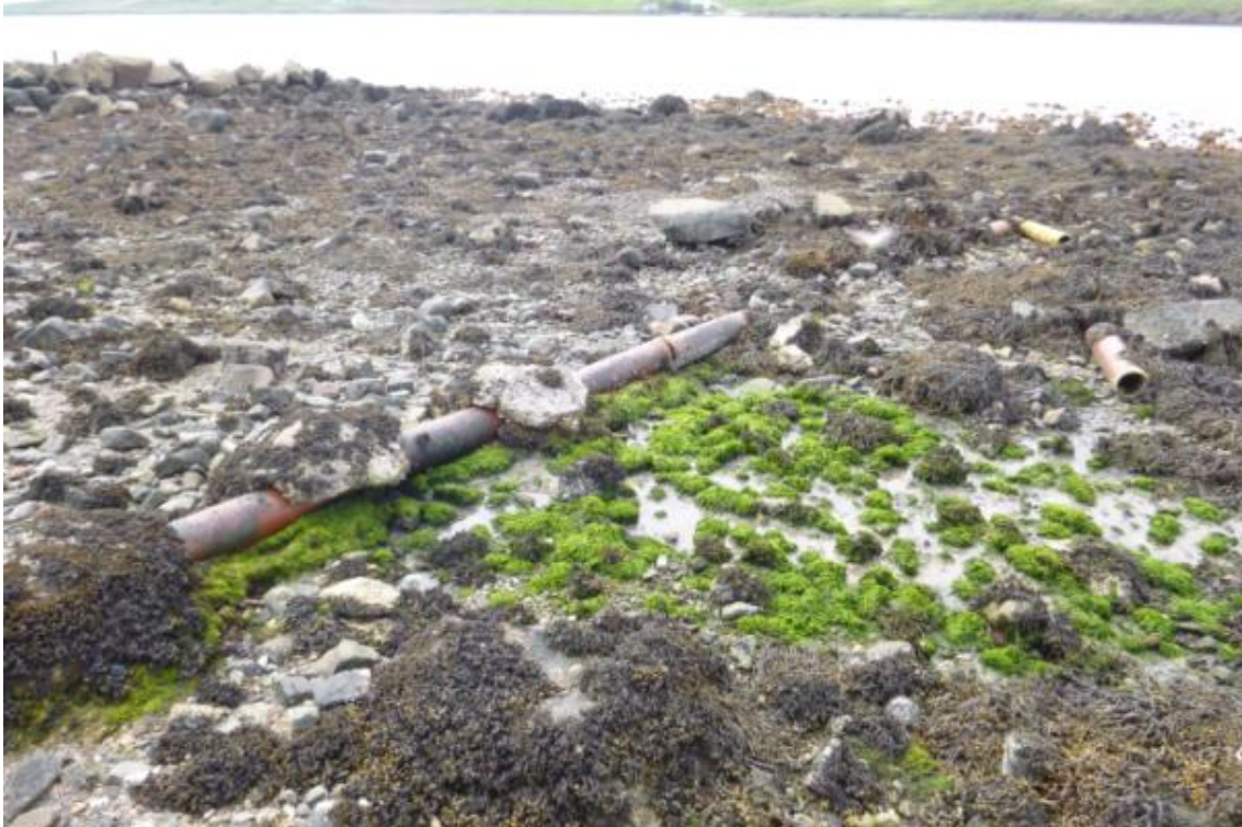
Figure 11 – Broken pipe with a grey discharge associated with a septic tank below a house in Brae.
