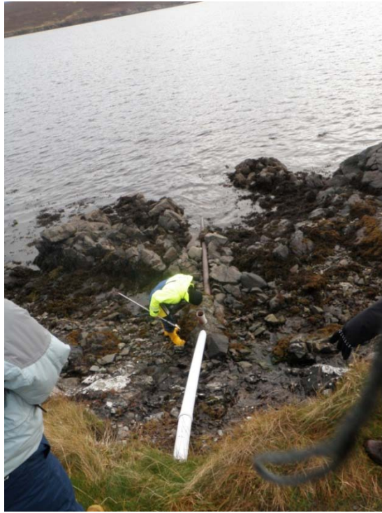
Figure 12 – Assessing water flow in a pipe discharging to the sea between the Greentaing and Buddascord fisheries.
