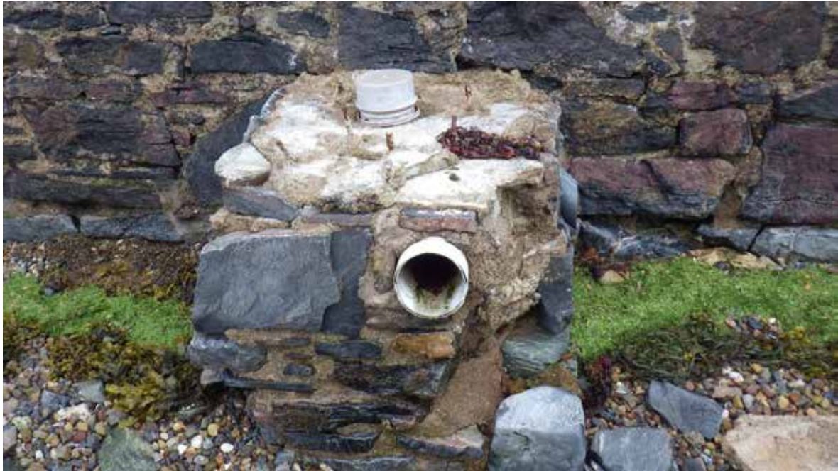
Figure 5: Discharge pipes on shoreline at Lower Askomill Road (Waypoint 17)
