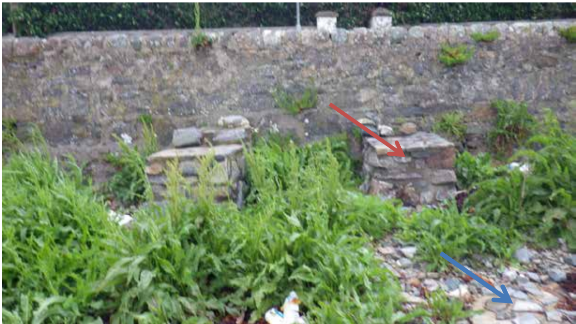
Figure 6: Example of tied-in sewage discharge pipe along the shore side of Lower Askomill Road (red arrow) with concrete infill on foreshore (blue arrow). (Waypoint 19)
