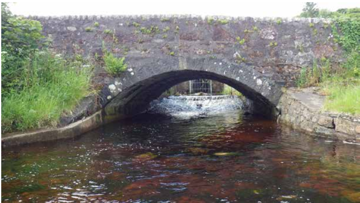
Figure 16: Glenramskill Burn, with unidentified discharge pipe on right shore next to bridge wall. (Waypoint 61)
