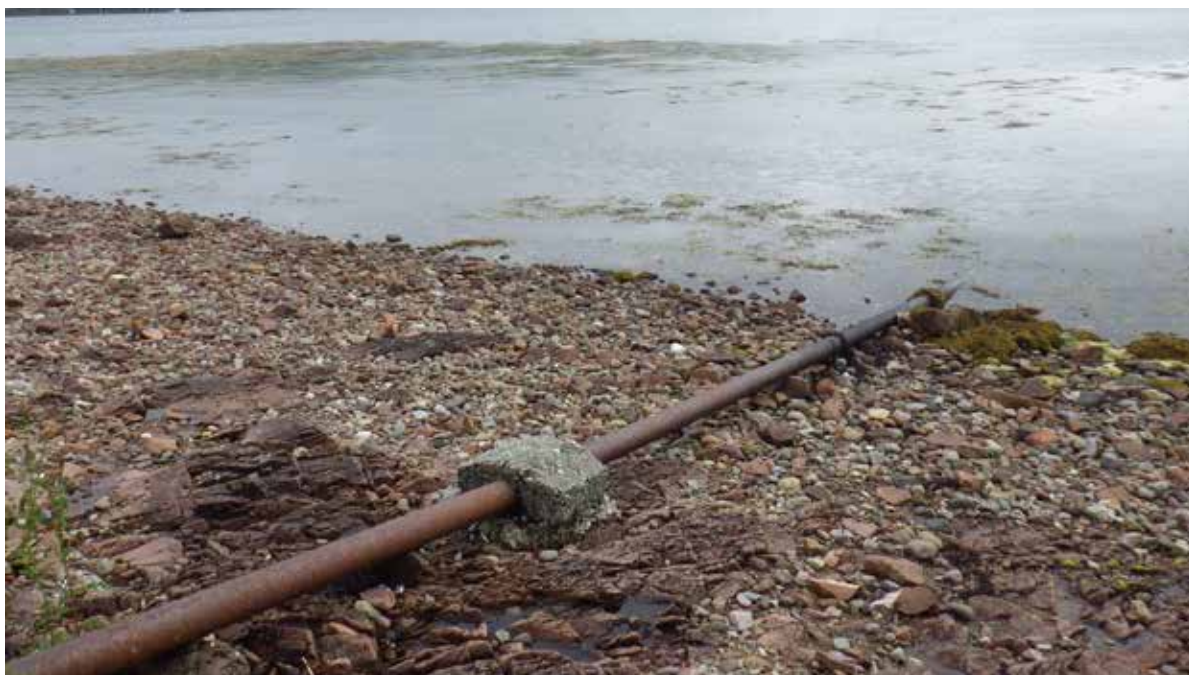
Figure 13: Typical discharge pipe running into Campbeltown Loch from shore in Kilkerran. (Waypoint 44)
