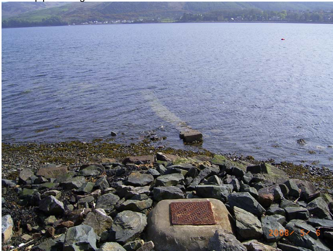
Figure 10. Inspection cover on north shore sewage pipeline with possible concrete pipe casing to sea behind.
