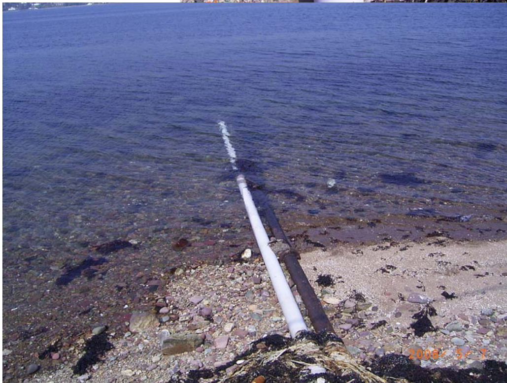
Figure 18. Private sewage discharge
