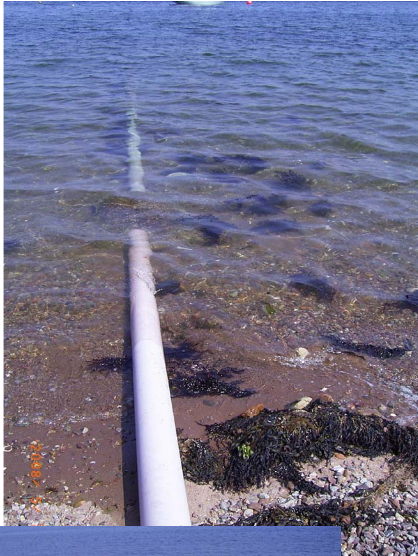
Figure 17. Private sewage discharge
