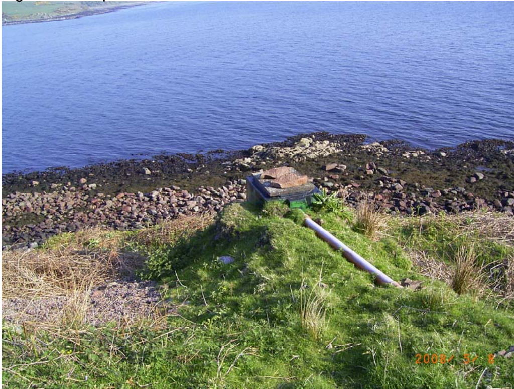
Figure 21. Septic tank on Davaar Island
