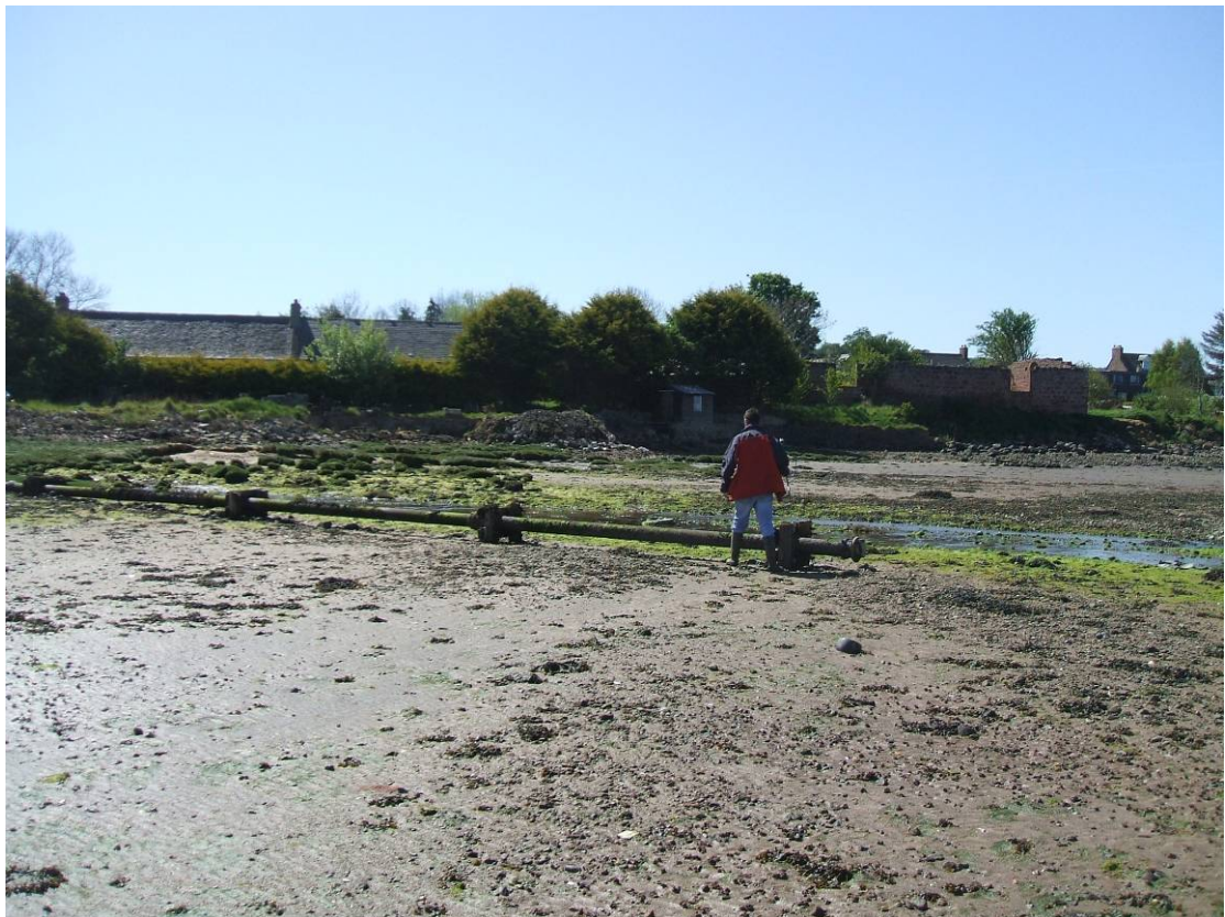
Figure 9. Jemimaville STW overflow
