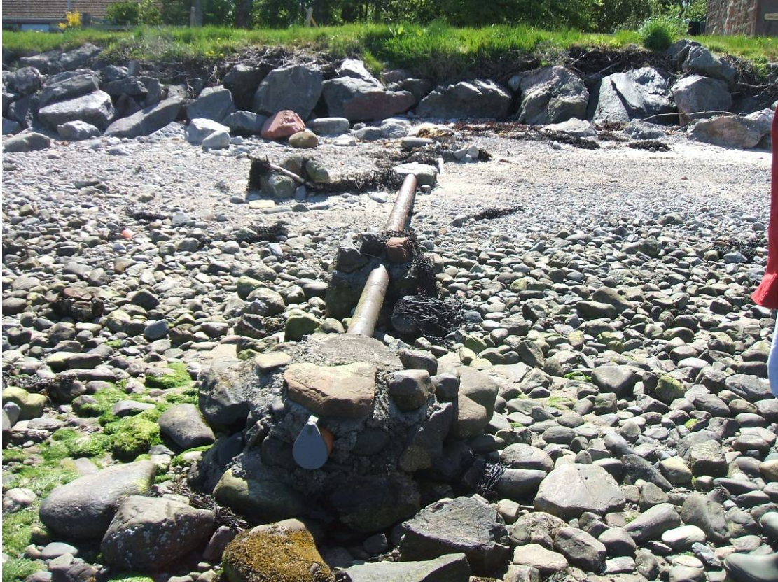
Figure 10 Discharge pipe at Balblair
