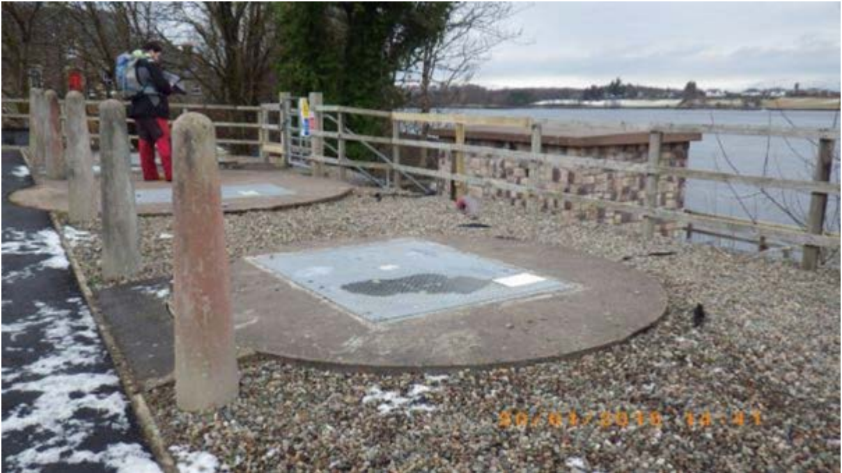
Figure 19. Scottish Water WWPS, Connel village, east of the south end of Connel Bridge. Waypoint 95.
