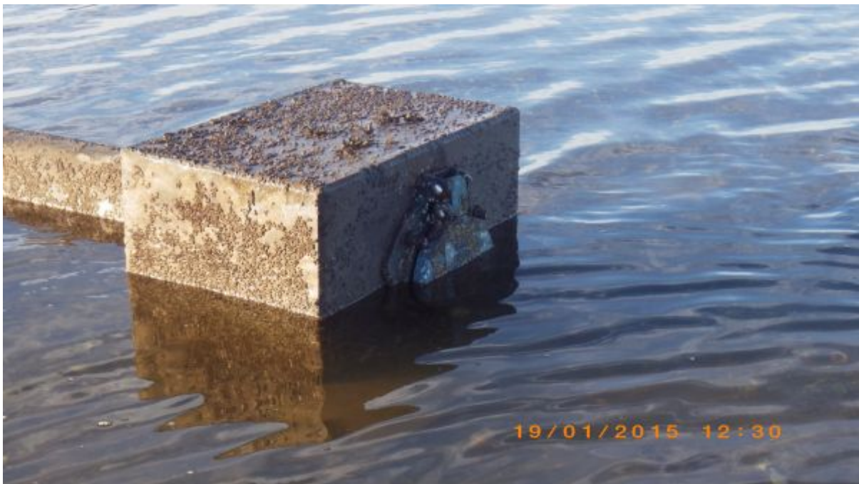
Figure 8. Dunbeg combined waste water overflow pipe end. Waypoint 16.
