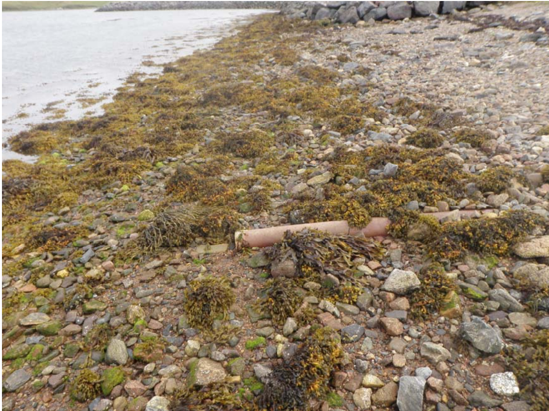
Figure 10. Discharge pipe running from pumping station across shore.
