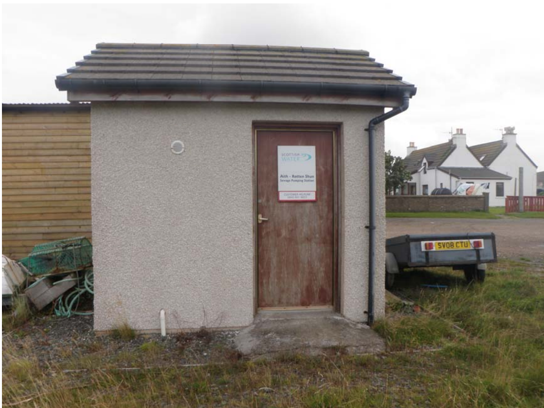
Figure 9. Aith - Rotten Shun sewage pumping station.
