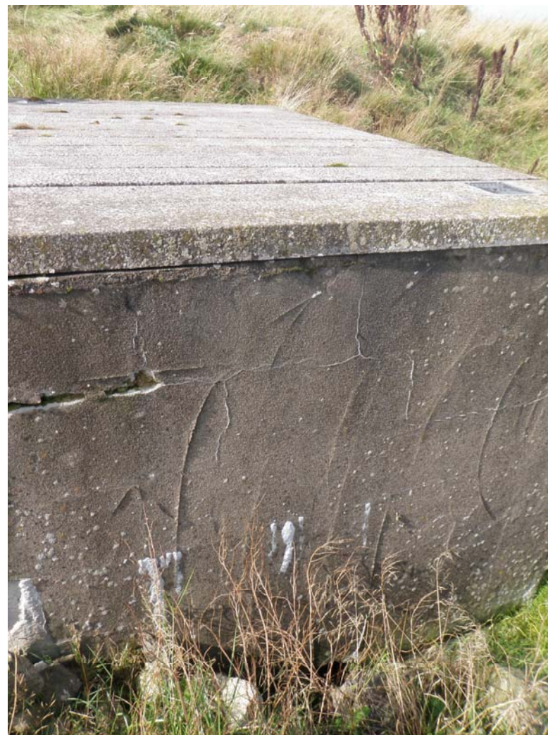
Figure 16. Septic tank with no discharge pipe, leaking at base.
