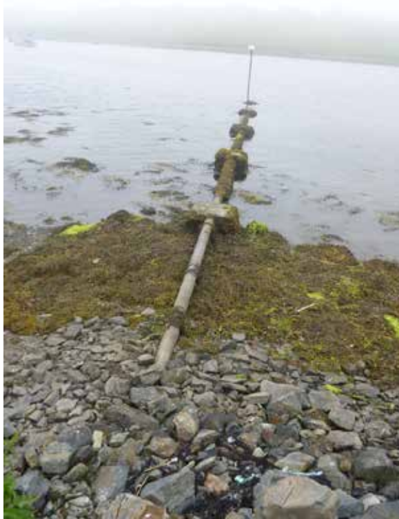
Figure 8 – Pipe associated with the Blydoit Sewage Pumping Station
