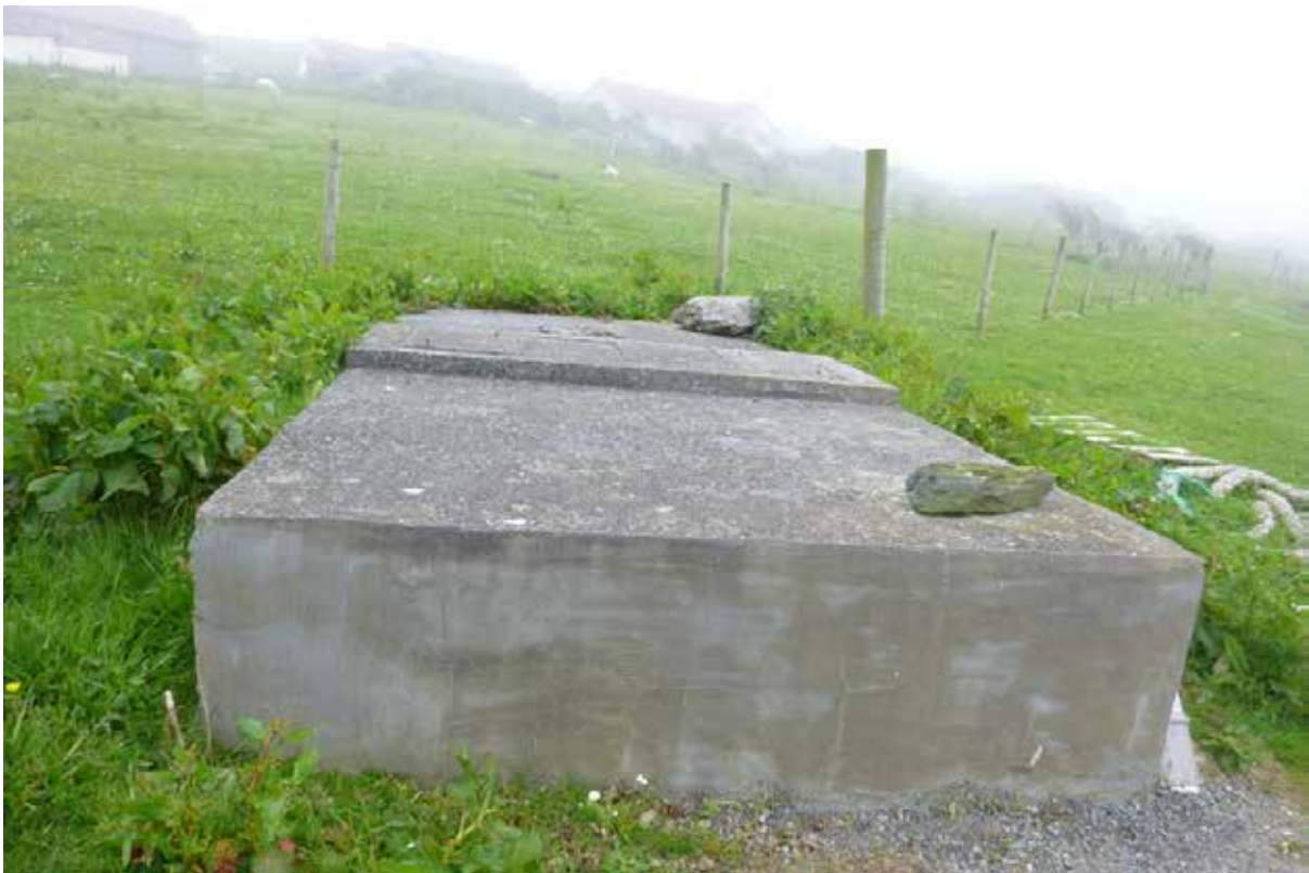
Figure 13 – Concrete septic at Cauldhame.
