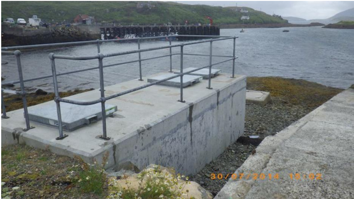
Fig. 11 Scottish Water communal septic tank Scalpay harbour north. Waypoint 38.
