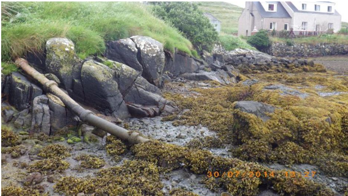
Figure 6. Broken and disused outfall pipe Ceann a Bhaigh, Scalpay. Waypoint 21.
