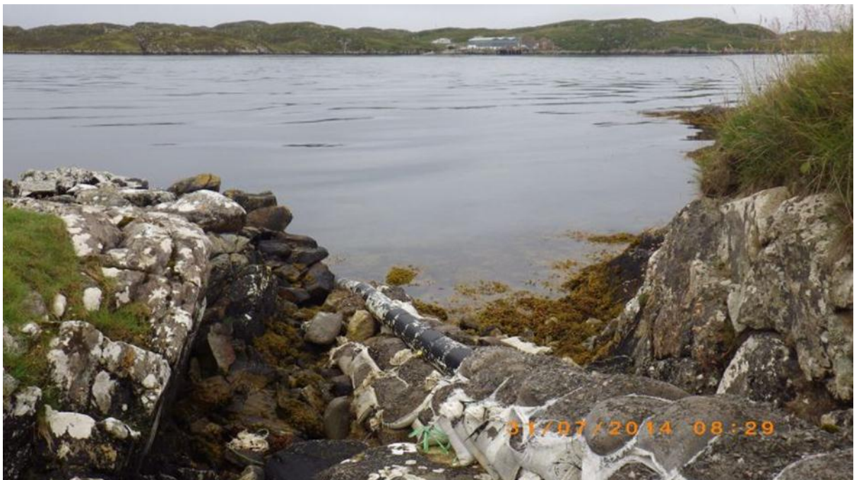
Fig. 14 Outfall pipe of 150 mm black plastic secured by bags of cement aggregate. Pipe end underwater. Waypoint 51.
