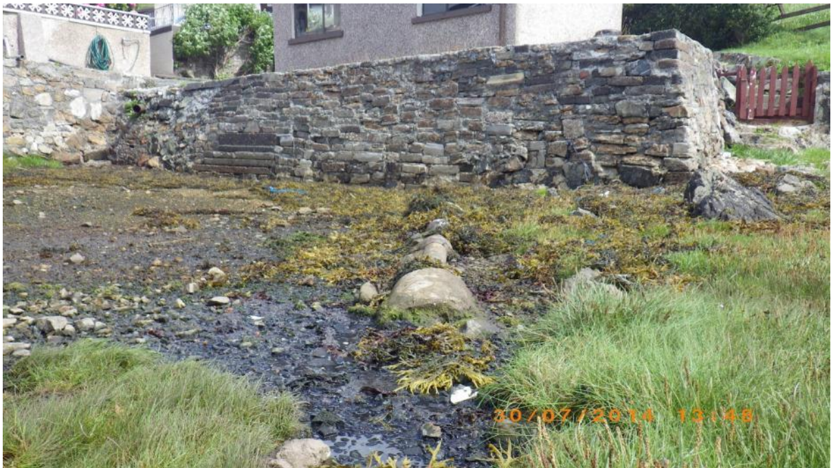
Figure 8. Stagnant but active ceramic outfall pipe. Waypoint 27.
