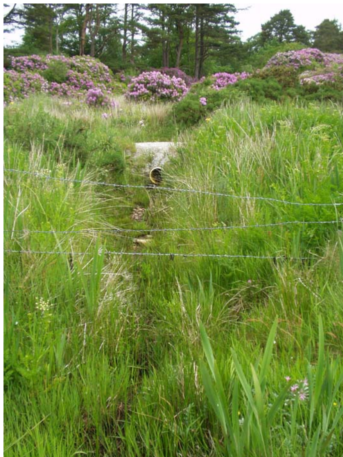
Figure 6. Drainage pipe under road, not flowing
