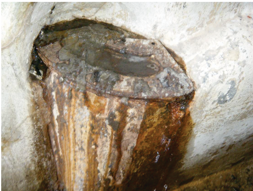
Figure 11. Foul discharge from metal plate
