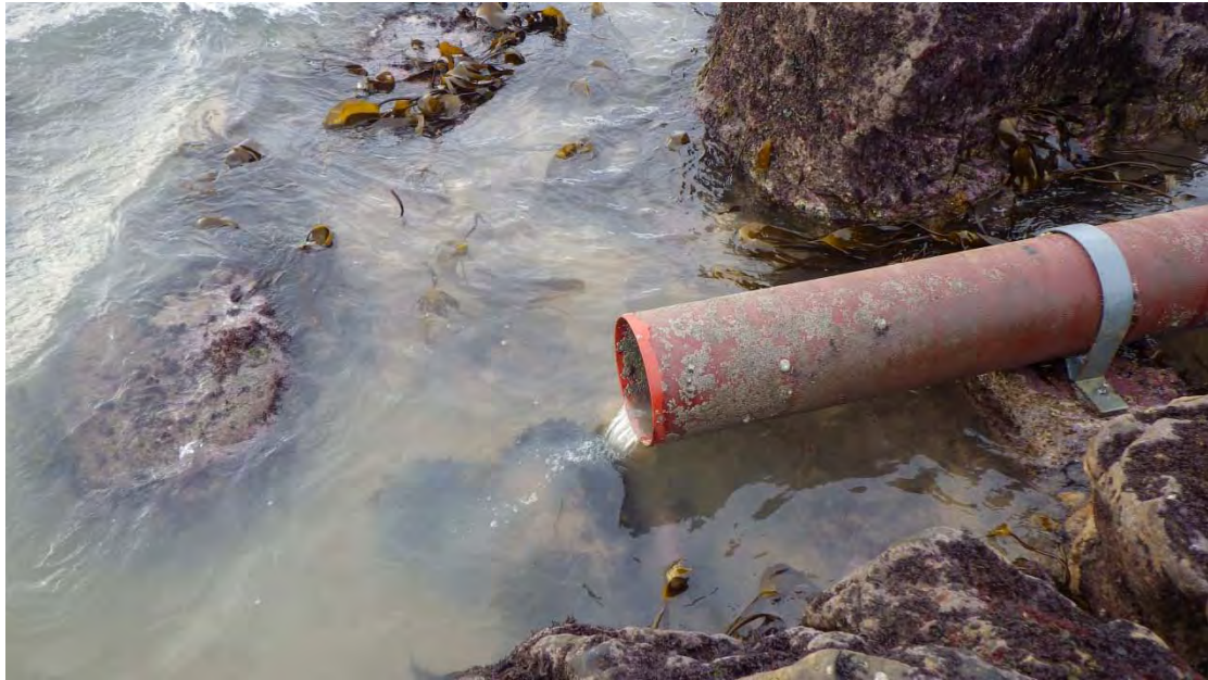
Figure 32. Plastic discharge pipe (Waypoint 33, ANS17)
