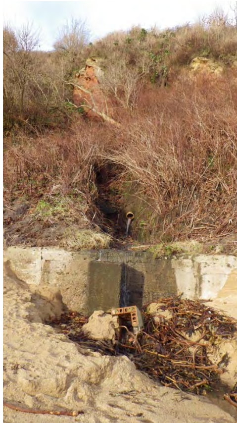
Figure 35. Stream or possibly discharge running downhill through pipe. The pipe is broken above beach, water/discharge running freely into sand (Waypoint 36, ANS19)
