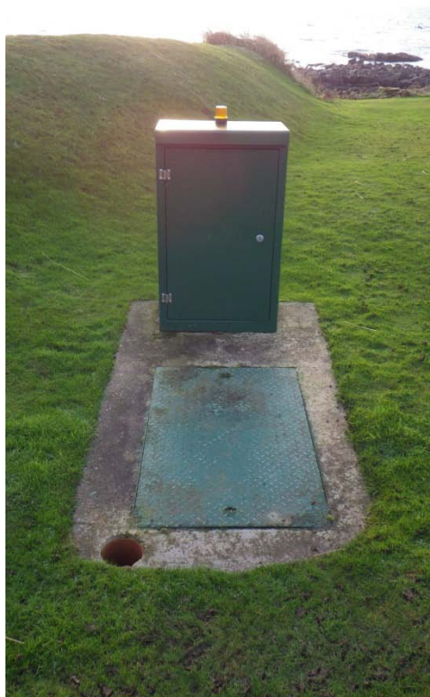
Figure 27. Manhole and electrical switchbox, in Sauchope Link Caravan Park, just outside Crail to the east (Waypoint 21)
