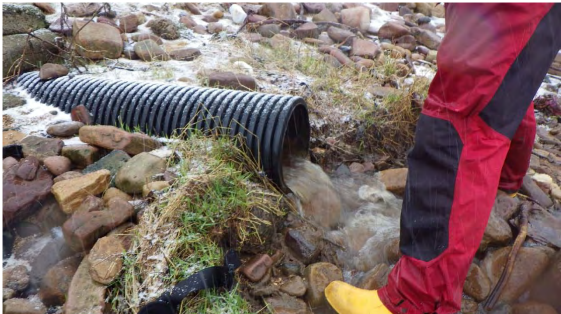
Figure 23. Large plastic outfall pipe by pig farm (Waypoint 17, ANS8)
