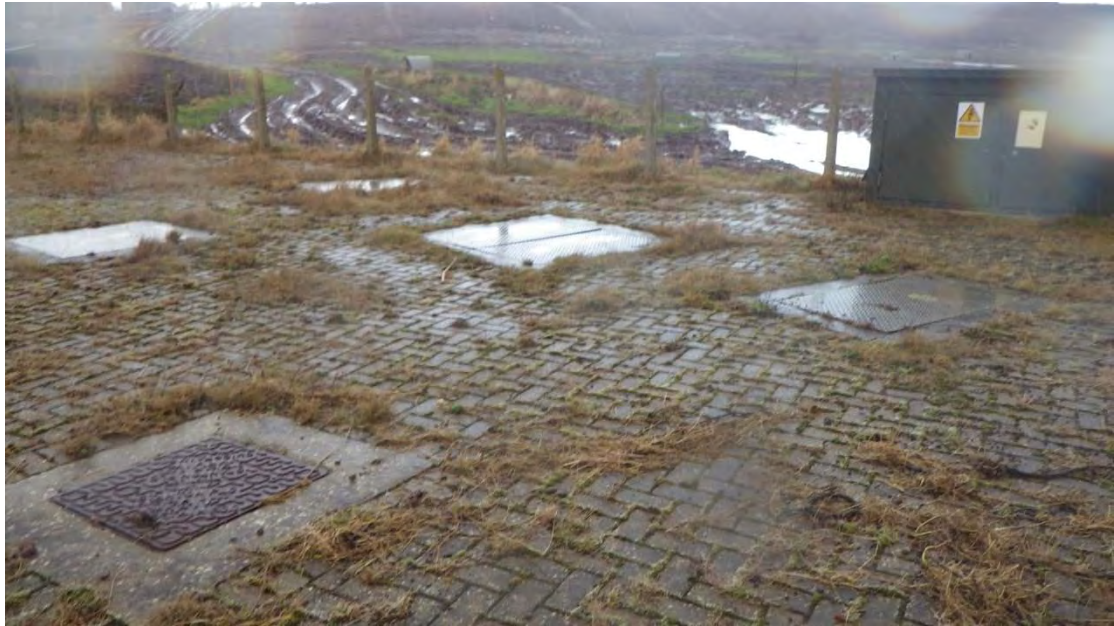
Figure 16. Sewage collection chamber at pig farm/caravan site (Waypoint 13)
