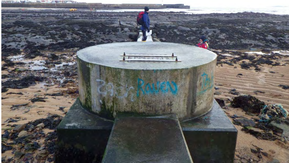
Figure 4. Sewage outfall pipe in Anstruther bay (WP2)
