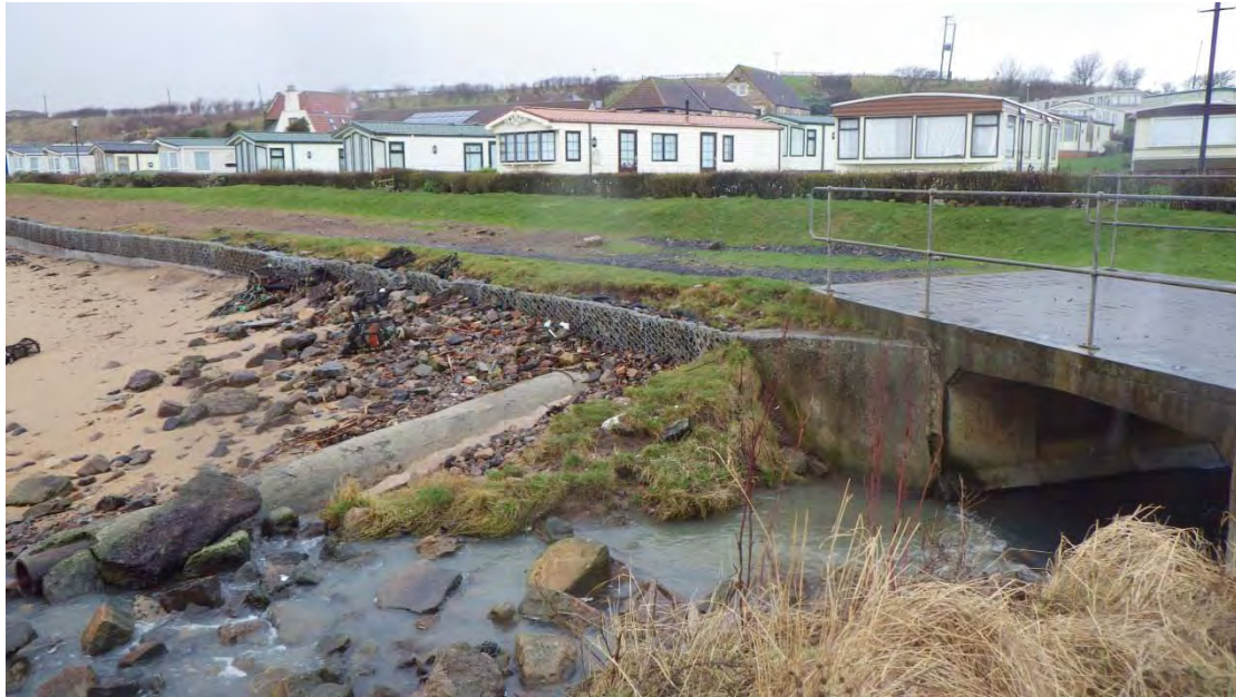
Figure 18. Old concrete outfall pipe next to sampled burn with no visible discharge (Waypoint 13)
