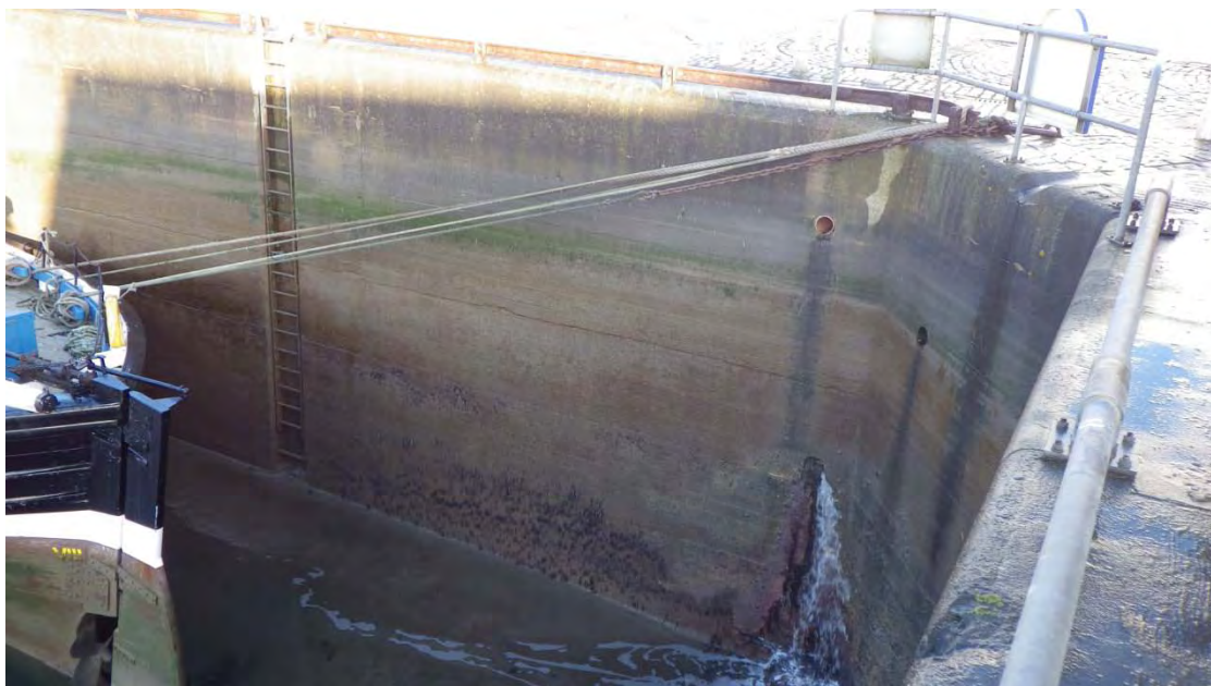
Figure 13. Discharge from harbour wall (Waypoint 8)
