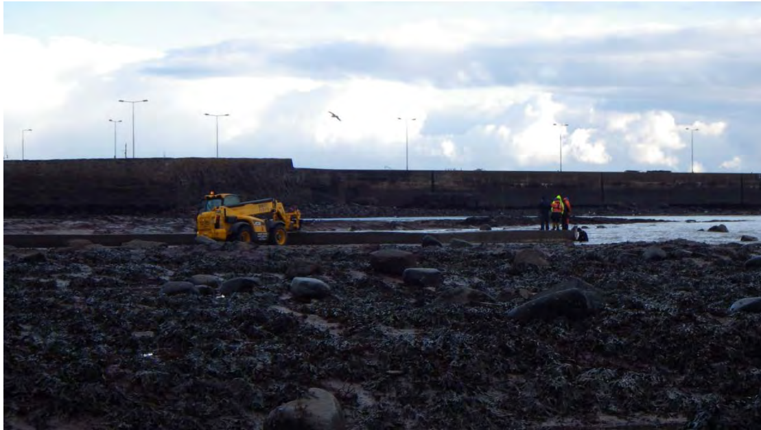
Figure 8. Concrete sewage pipe running into bay. Workers fitting a large hood at the end (Waypoint 4)
