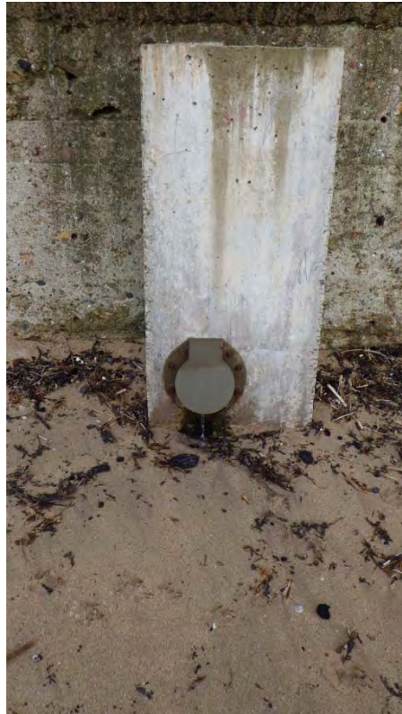
Figure 34. Discharge from lidded valve on beach by Crail harbour (Waypoint 35, ANS18)
