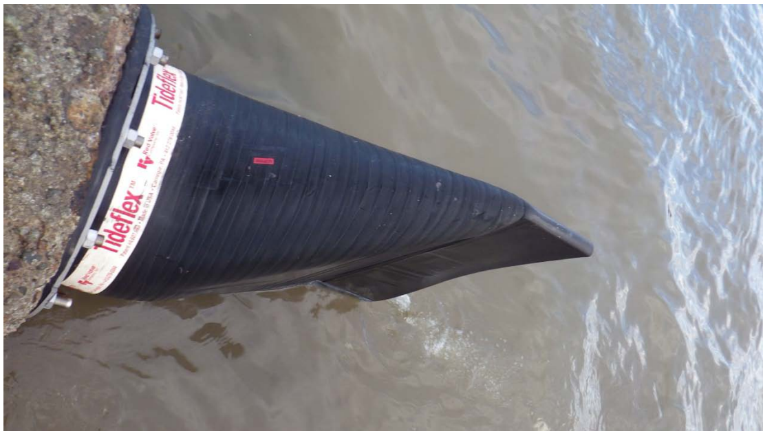
Figure 9. The end of concrete sewage pipe with fitted a large hood at the end (Waypoint 4)
