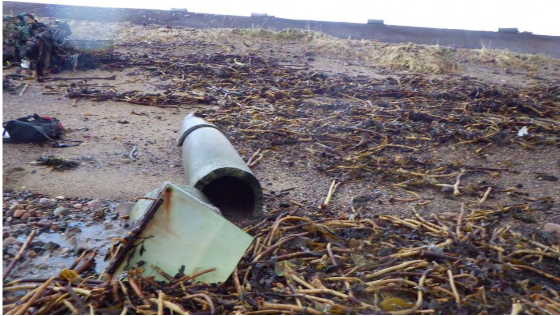
Figure 20. Broken outfall pipe by pig farm discharging onto shore (Waypoint 15, ANS7)
