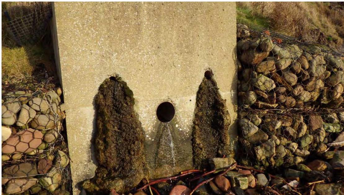
Figure 29. Discharge on beach, cement block with 3 discharge pipes (Waypoint 26, ANS14)
