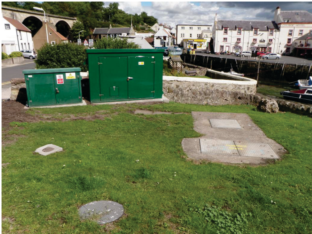
Figure 25. 5 inspection covers and 2 large green units, possible pumping station, no signage
