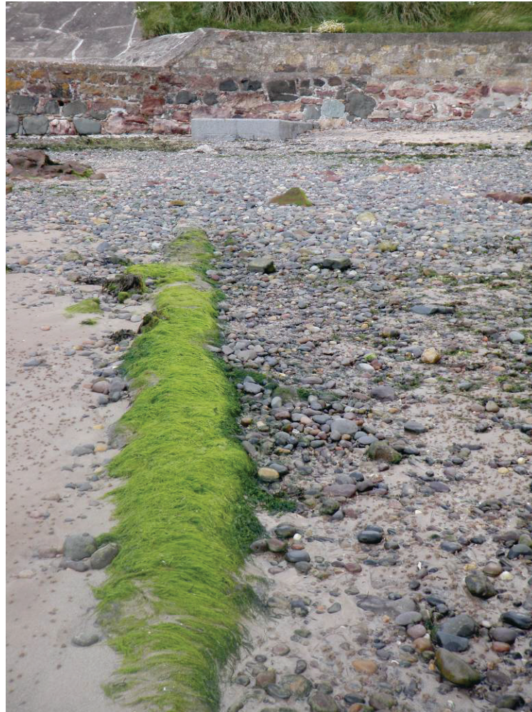
Figure 24. Septic tank and outfall pipe covered in green algae, could not locate end of pipe
