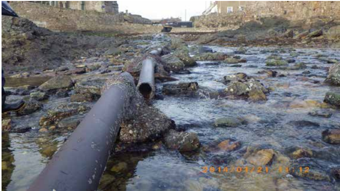
Figure 9. Iron pipe broken with no flow follows the Inverie Burn down to the shore. Associated with waypoint 17
