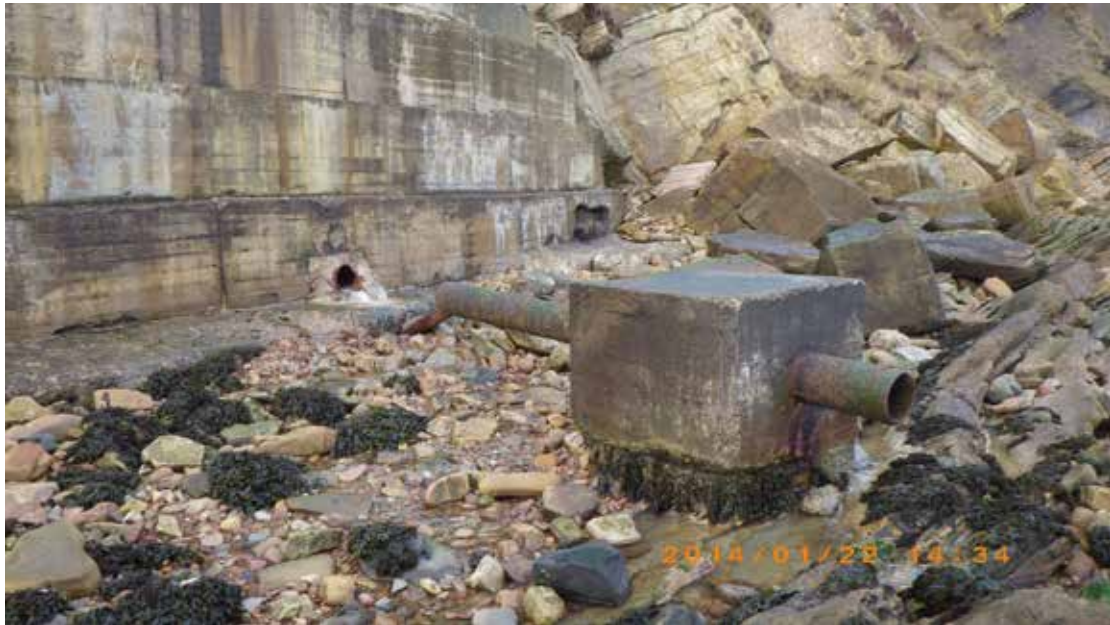
Figure 21. Pipe revisited from waypoint 65. Pipe is broken and flowing heavily. Associated with waypoints 65 & 68 and sample FWFEP8
