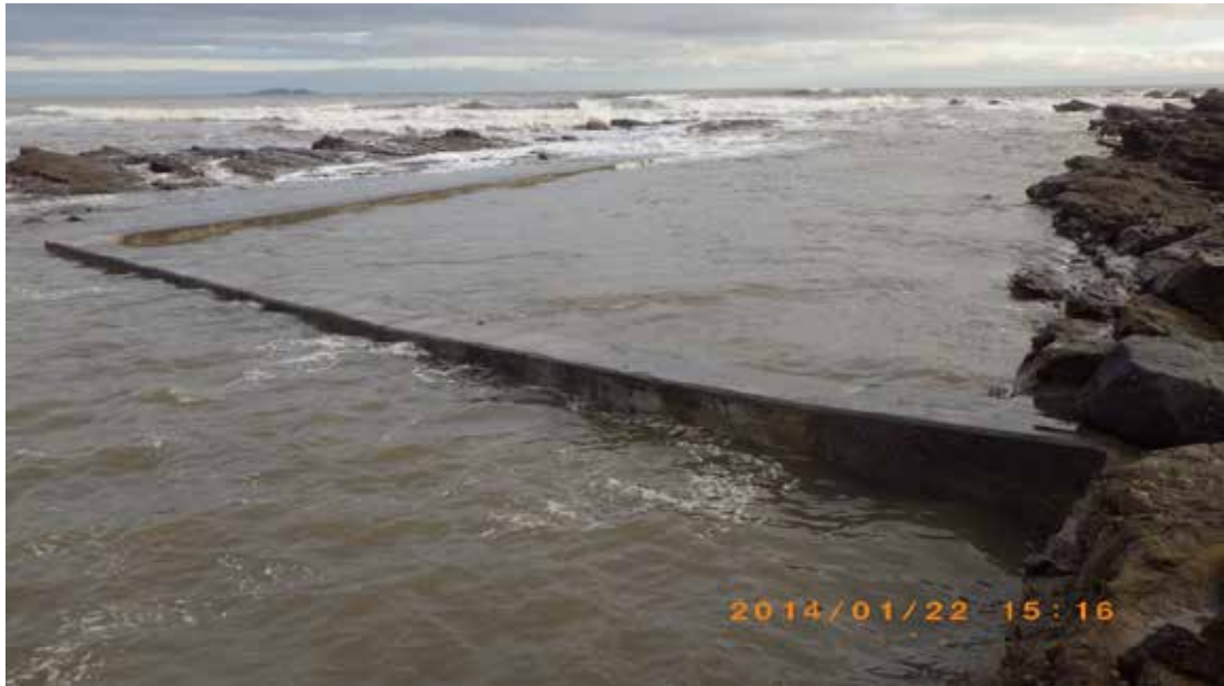
Figure 23. Concrete encased pipe going out to sea. Associated with waypoint 76 and sample SWFEP9
