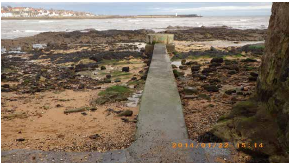
Figure 22. Large concrete structure with concrete encased pipe going out to sea. Associated with waypoint 75
