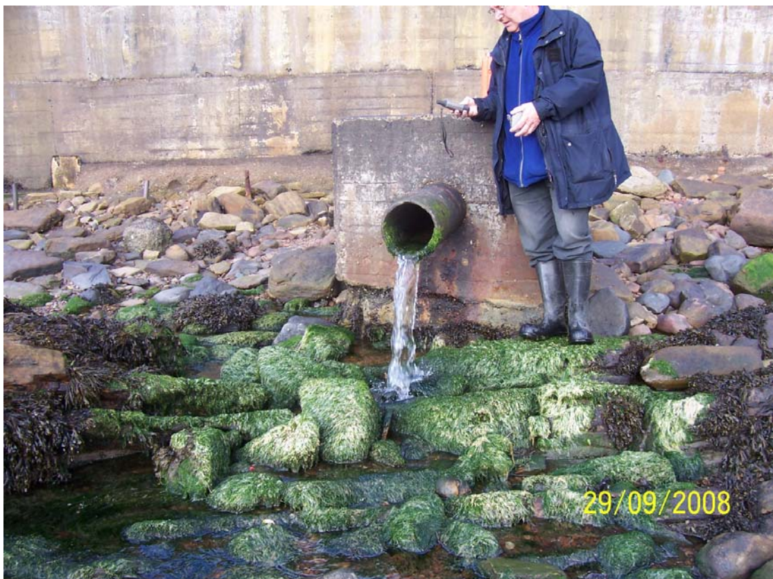
Figure 22. Outfall pipe (Water sample 5)
