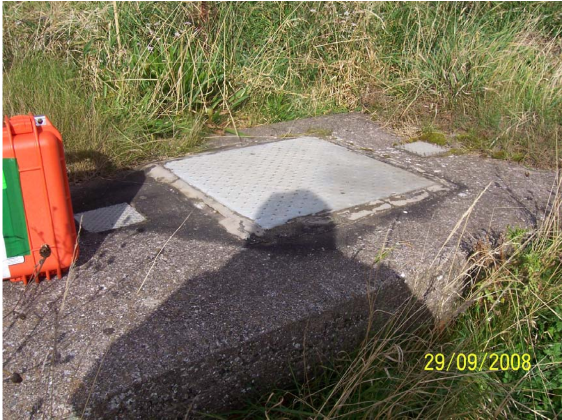
Figure 21. Manhole possibly connected to unknown building on golf course
