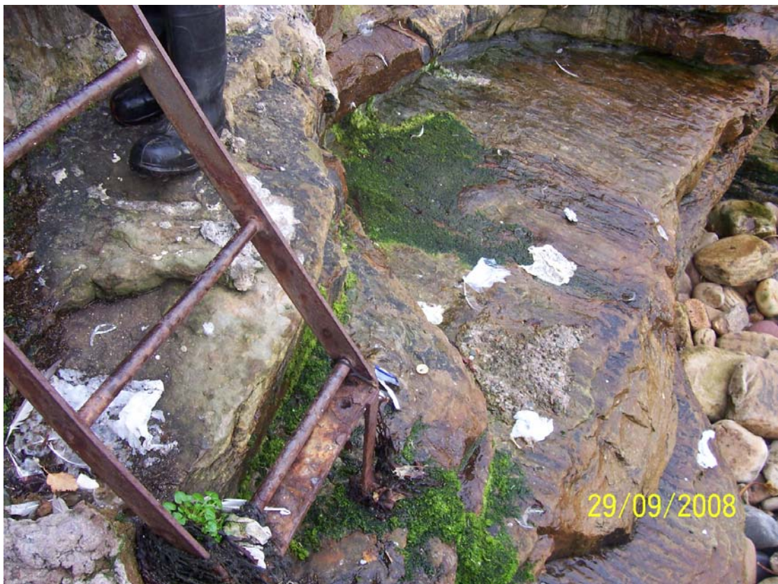
Figure 4. Evidence of sewage
