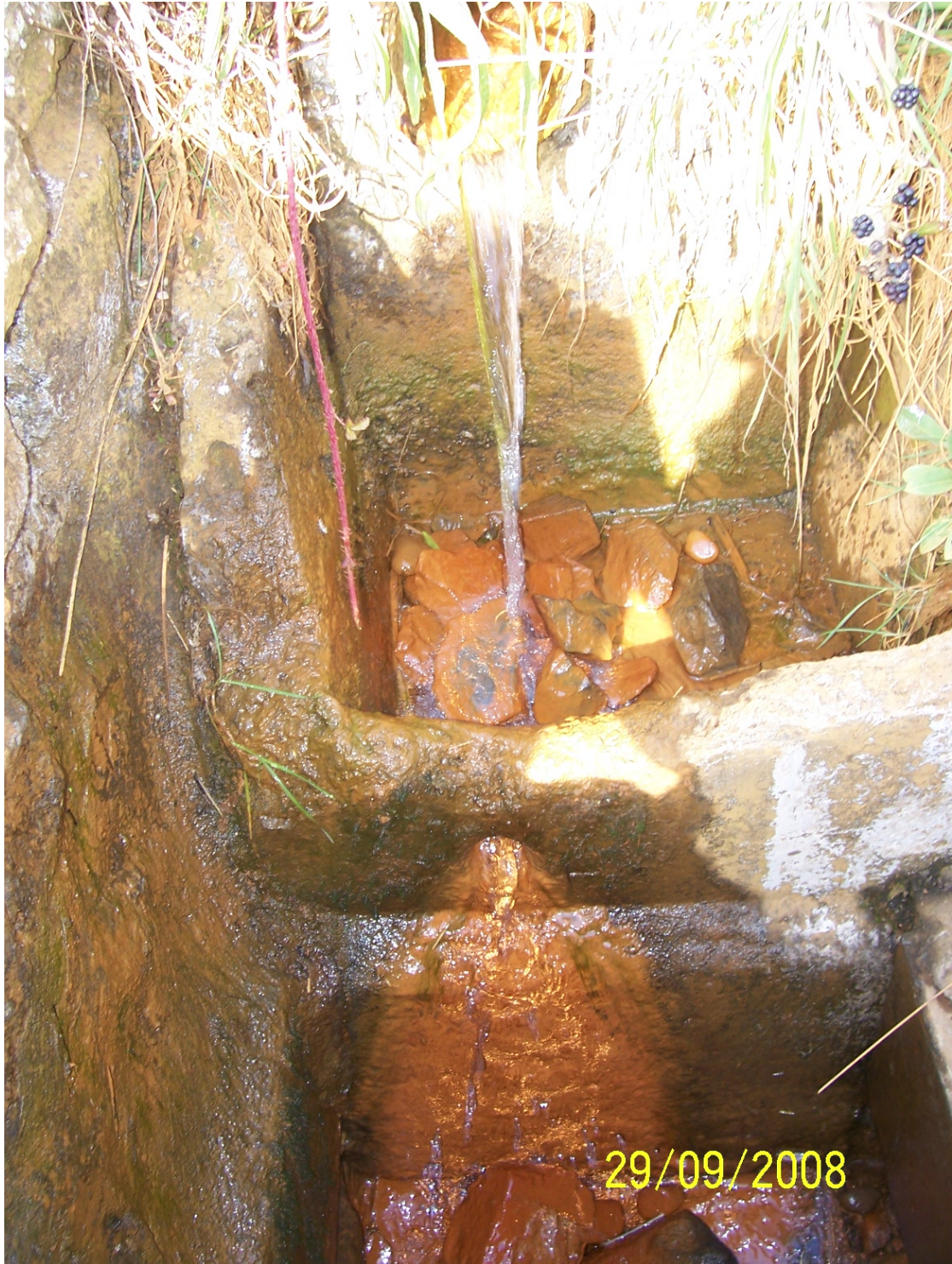
Figure 33. Outfall and seepage from Figure 44
