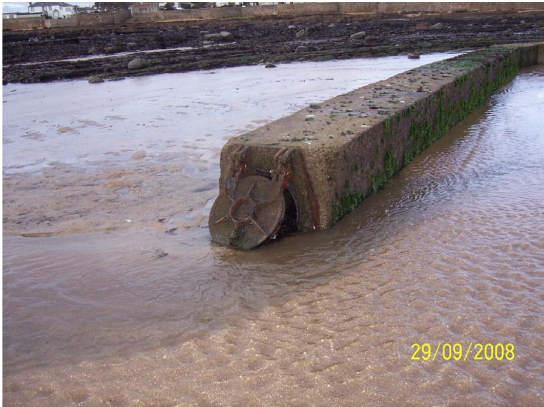
Figure 13. Unknown outfall (Water sample 9)
