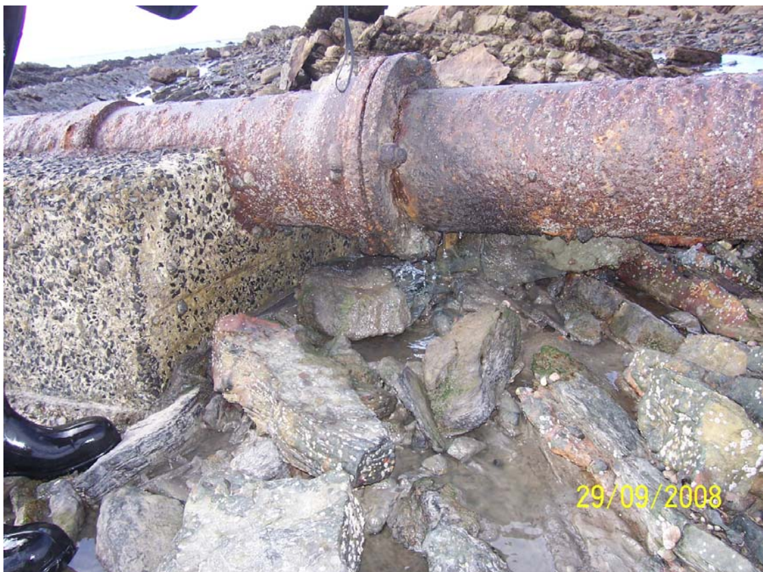
Figure 24. Outfall pipe (Figure 35) leaking, strong smell of sewage (Water sample 10 taken)
