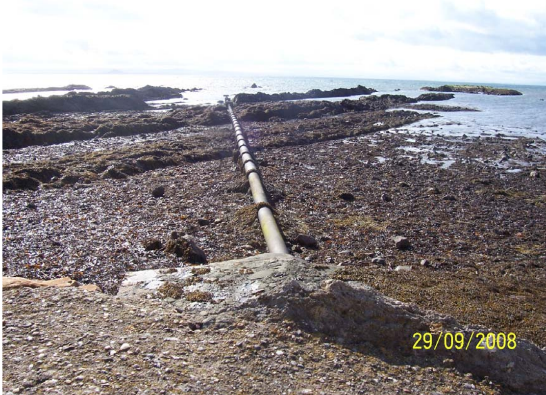
Figure 30. Pipeline believed to be overflow for a mid line pumping station that pumps sewage to the pumping station at Anstruther or St Monans
