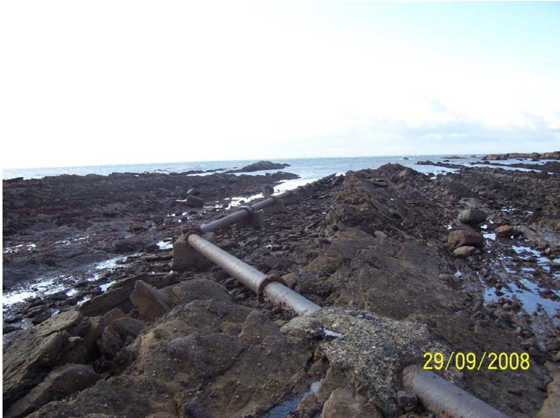
Figure 23. Outfall pipe running into the sea. End of outfall under water
