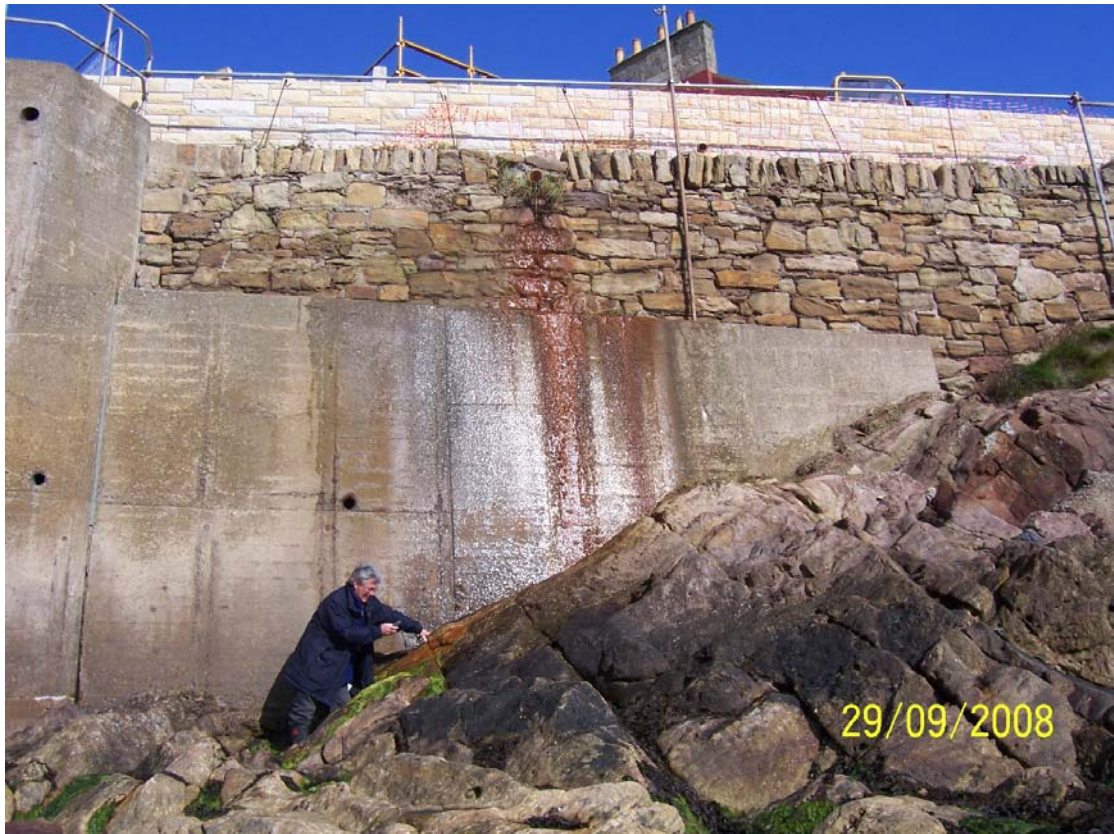
Figure 25. Location of outfall with seepage
