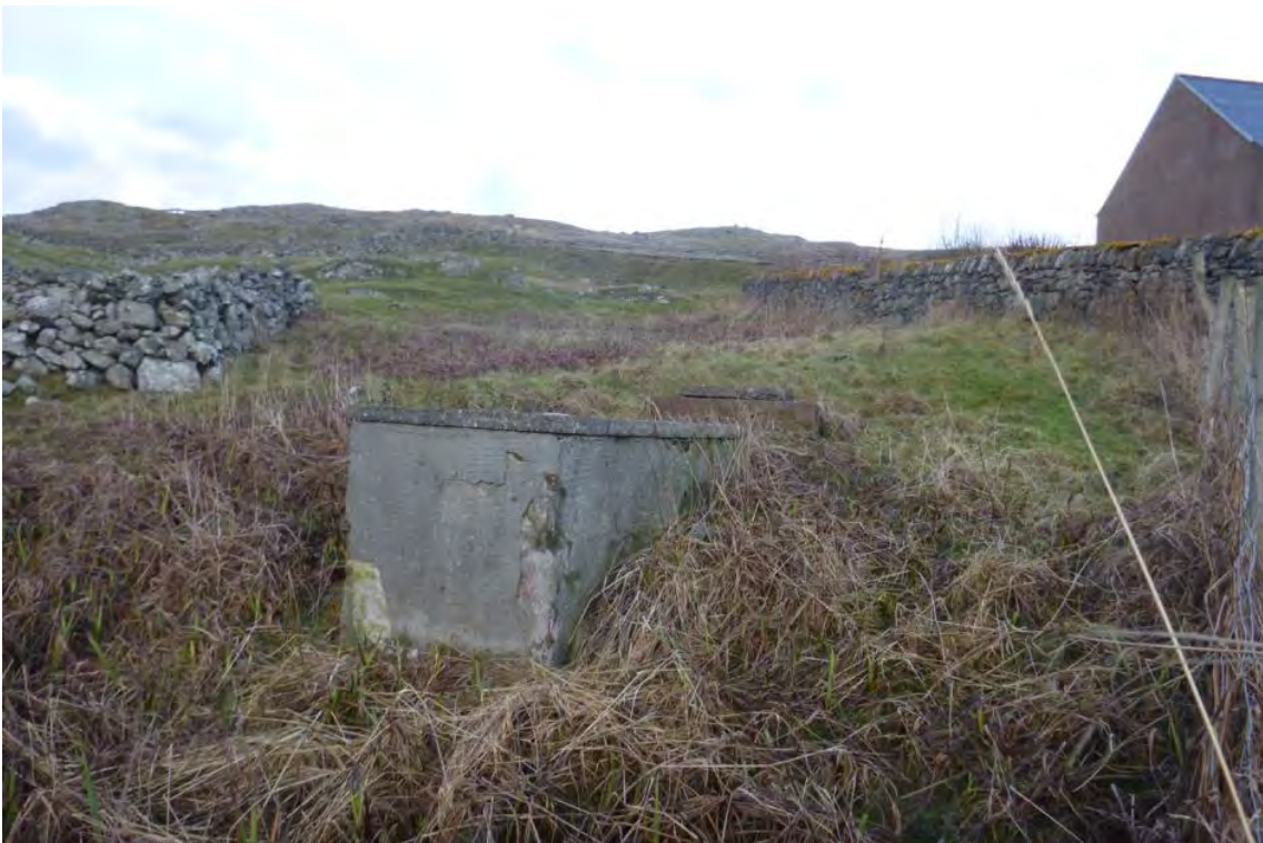
Figure 11 – Concrete septic tank associated with dwelling house and small community centre above.
