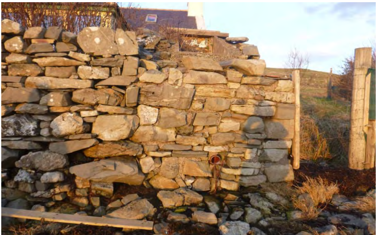
Figure 13 – Outlet pipe with no flow from dwelling house in close proximity to shoreline.
