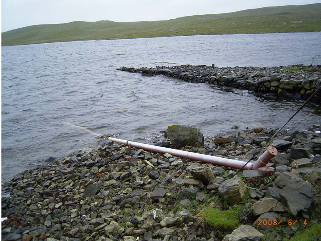
Figure 5. Wastewater discharge at Bridge of Walls
