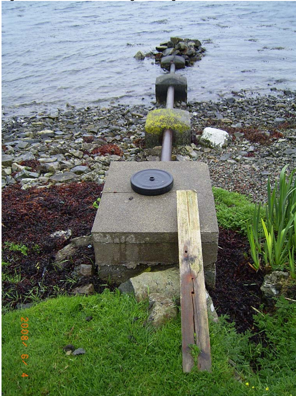
Figure 7. Wastewater discharge at Bridge of Walls
