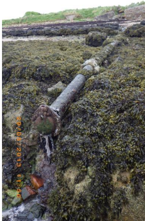
Figure 14. Freshwater sample (GPFW3) taken from pipe with raw sewage. Associated with waypoints 28 and 29.
