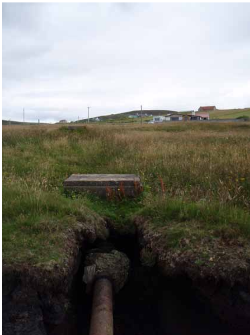
Figure 11. Septic tank joined on to outfall pipe shown in Figure 10
