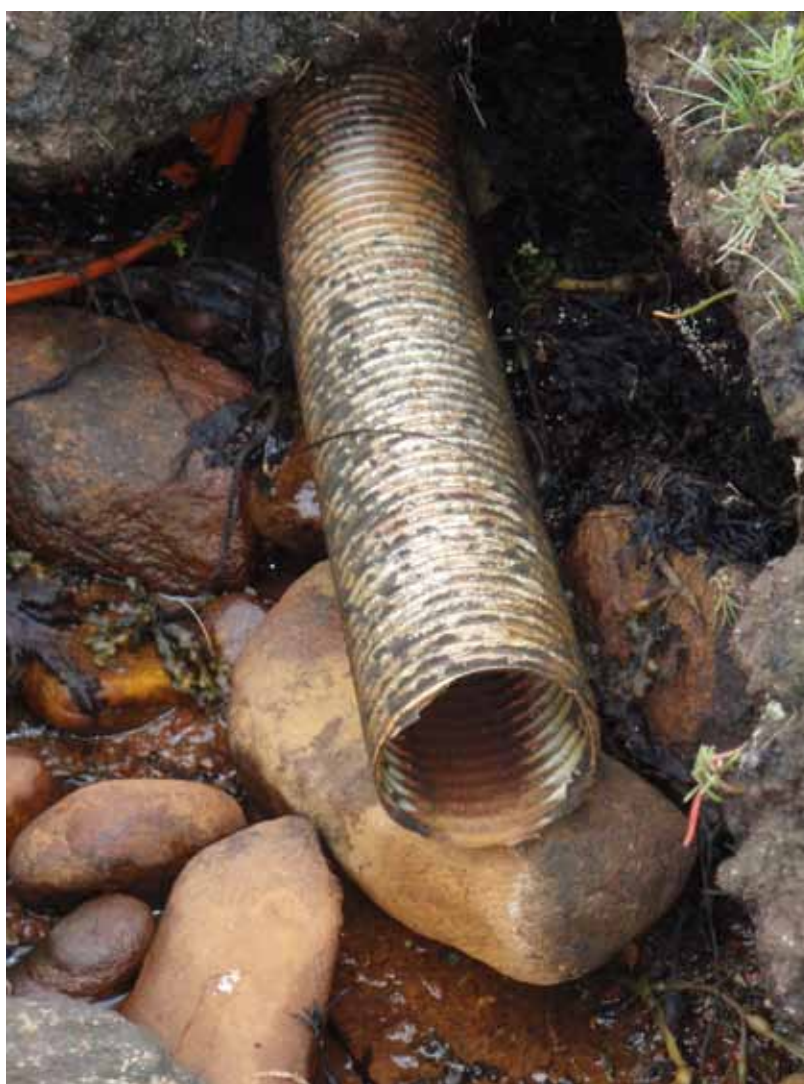
Figure 7. Outfall pipe, not flowing
