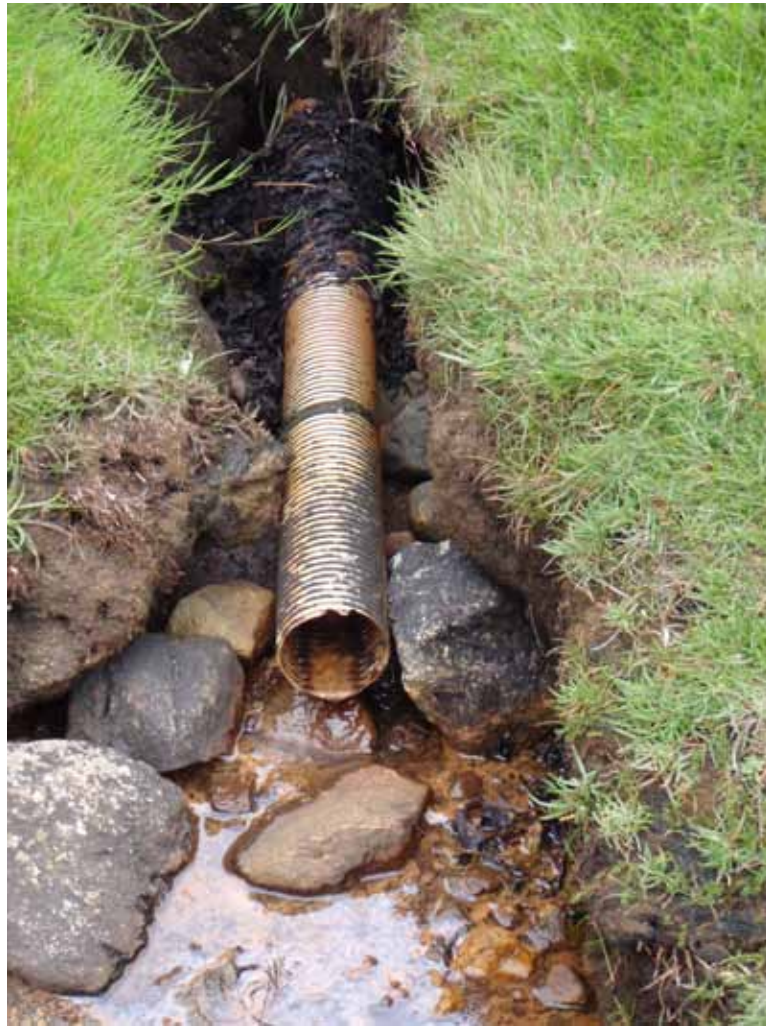
Figure 8. Outfall pipe, small flow, location of freshwater sample HVFW2
