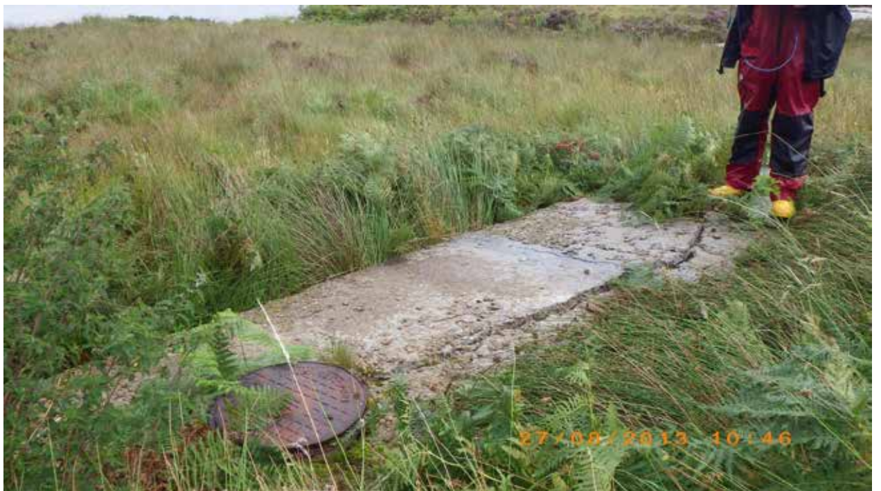
Figure 12: Septic tank for house on Aird Mhor peninsula with longitudinal crack through concrete. Waypoint 51.
