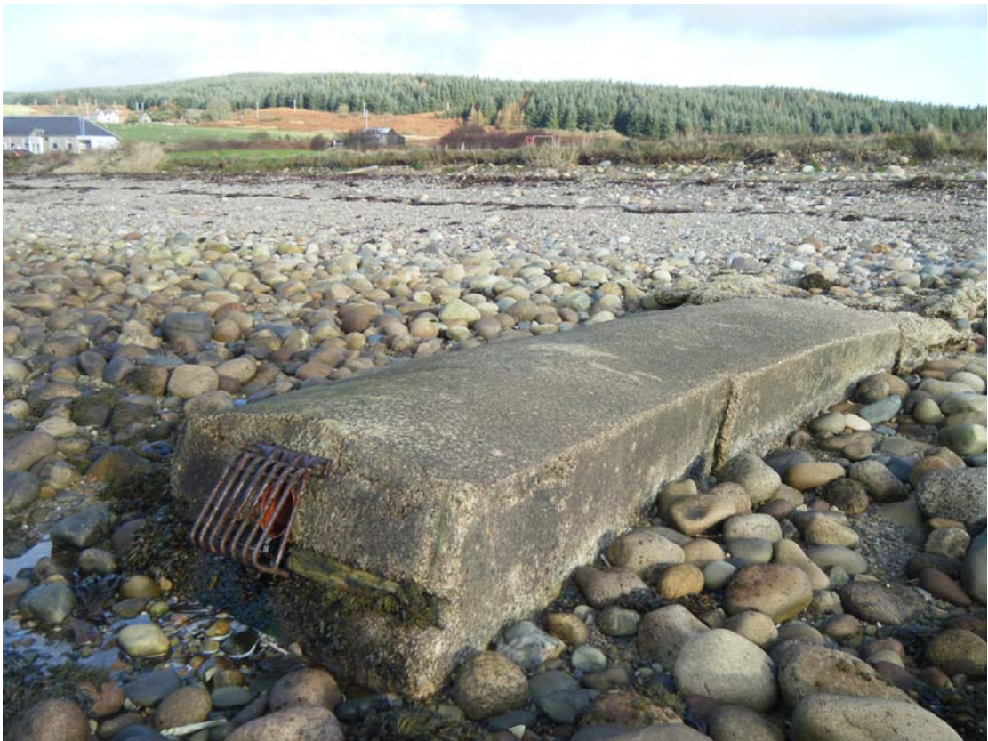
Figure 15. Concrete drainage pipe leading onto beach, possibly from golf course
