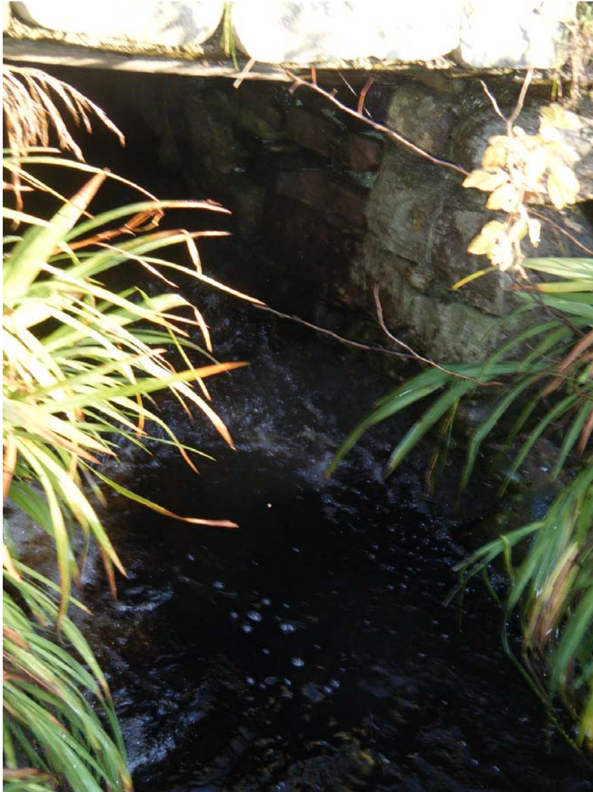
Figure 23. Culverted stream at school house water sample 14
