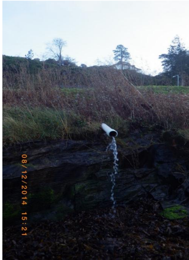
Fig 9. Pipe discharging water onto shore, unplanned freshwater sample KCFW4 taken, associated with waypoint 21.
