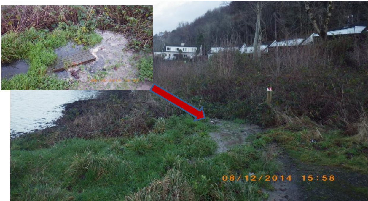
Fig 10. Houses at Dungallan Terrace with overflowing manhole. Insert shows raw sewage around manhole cover. Associated with waypoint 28 and location of contaminated freshwater sample KCFW6.
