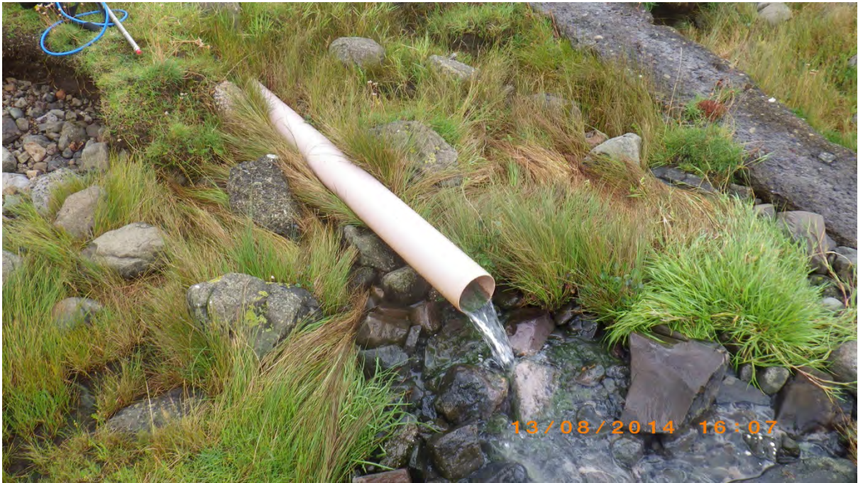
Figure 10: Pipe present below hotel at Tiroran, with active discharge (WP 26)
