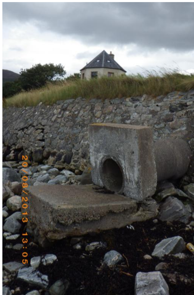
Figure 10. Concrete pipe protruding under road onto shore with a small round house behind. Associated with waypoint 21.
