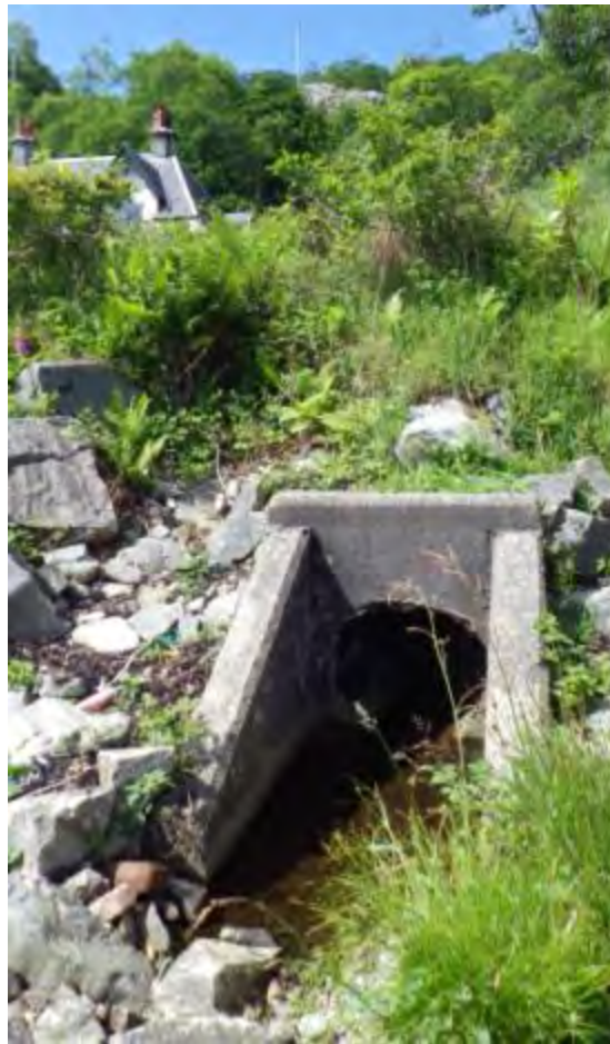
Figure 6. Culvert below house at Cuilidarrach. Associated with waypoints 13 and 14. Site of freshwater sample LBFW5.
