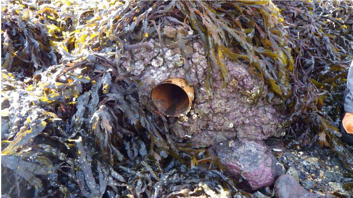
Figure 13. Sewage pipe running from house on shore into sea. Waypoint 12.
