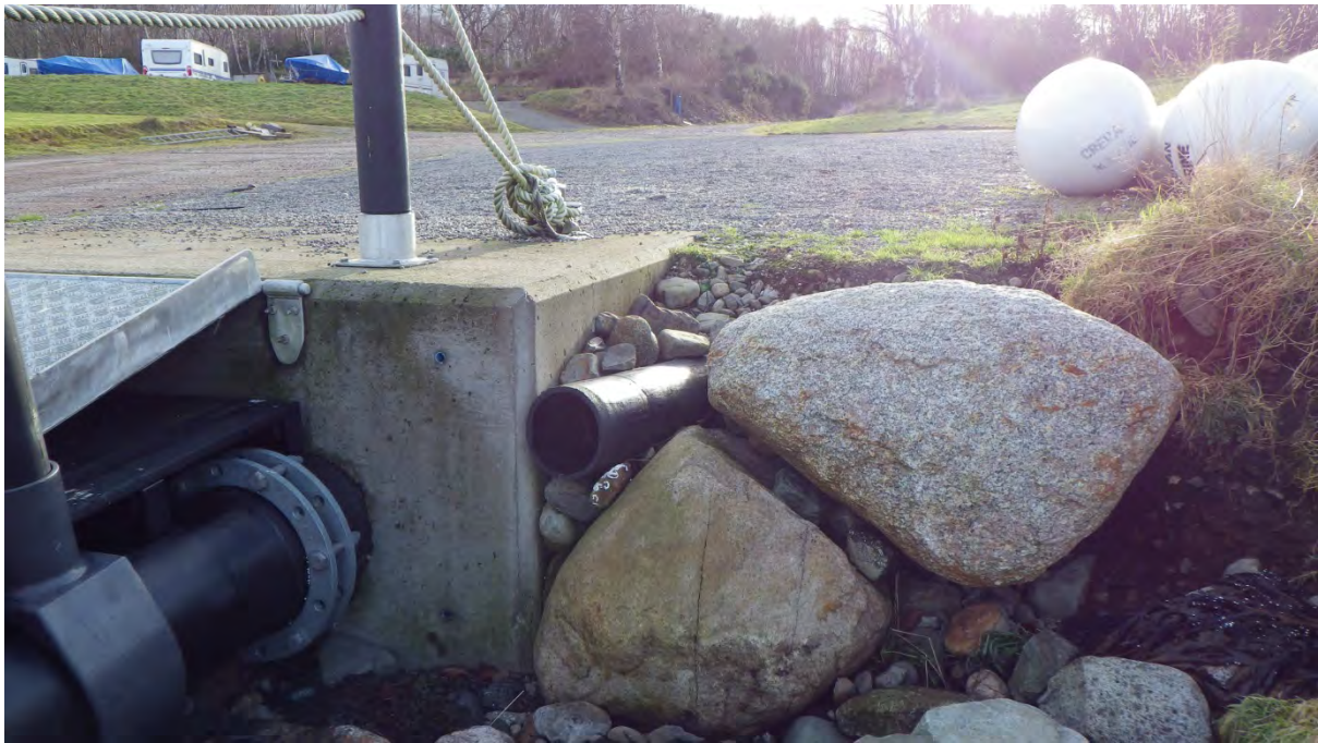
Figure 9. Plastic pipe with no discharge at pontoon by caravan park. Waypoint 5.
