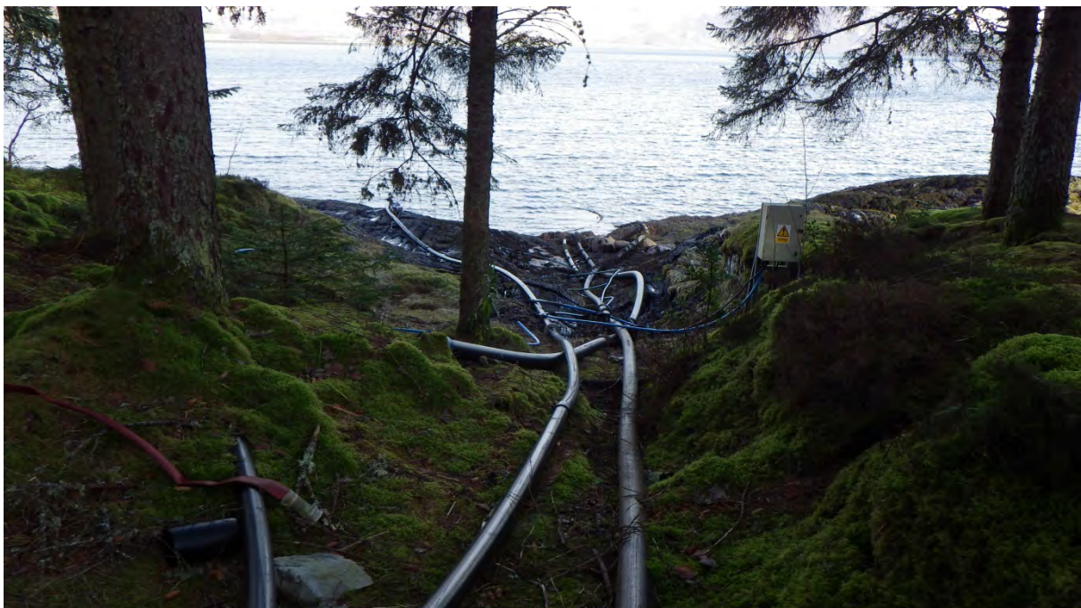
Figure 12. Pipes run up and down on shore next to SLC with pump attached near water. Waypoint 10.
