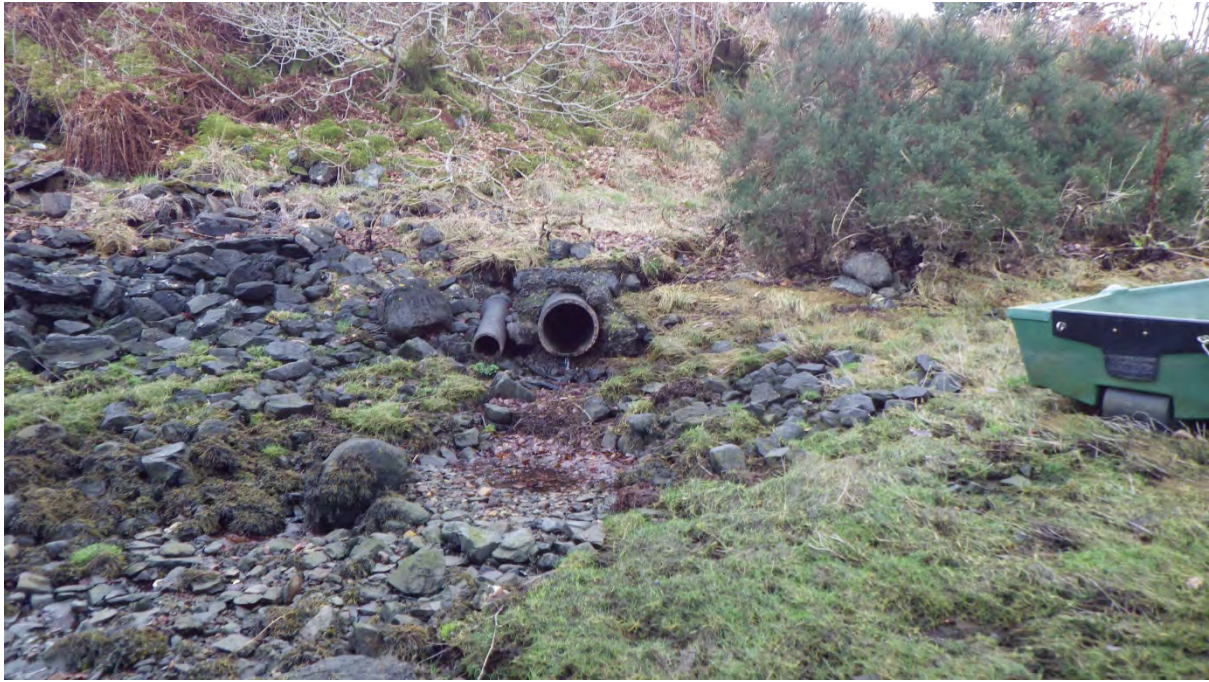
Figure 15. Clay pipes on shore next to house. Waypoint 20.
