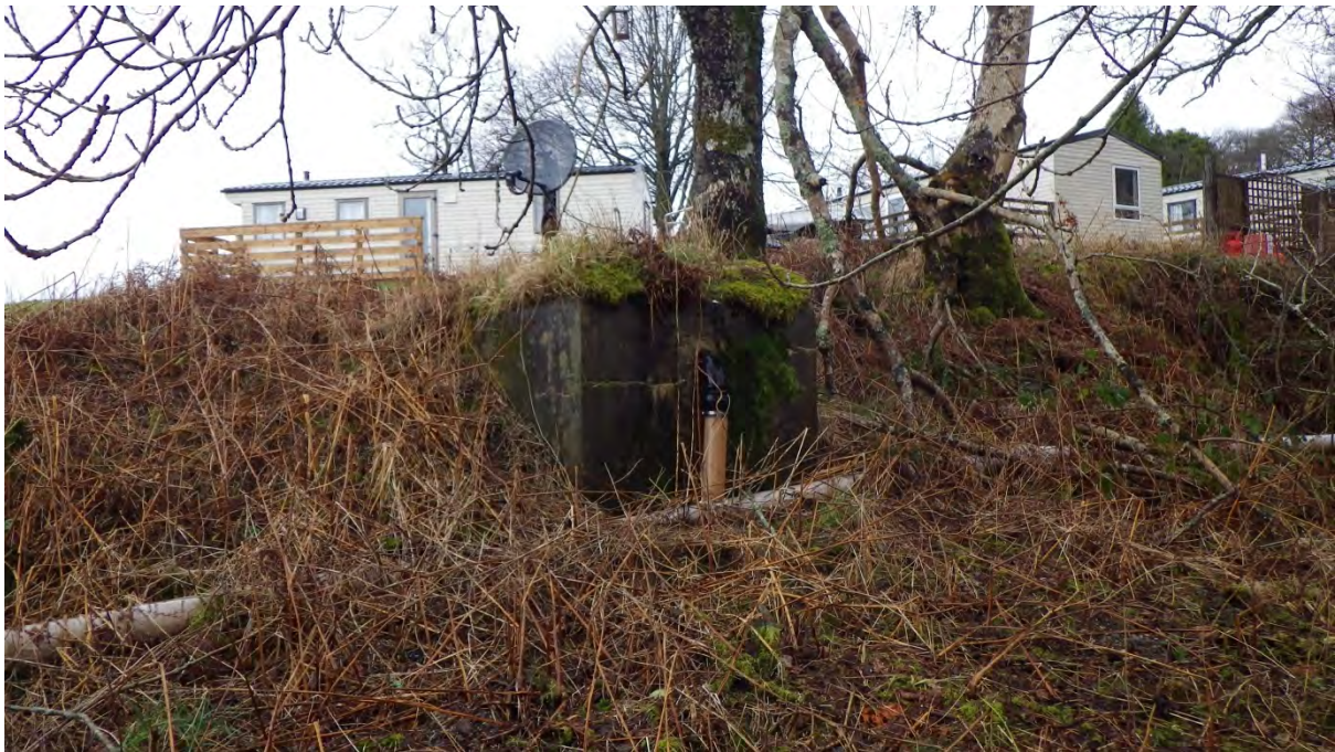
Figure 26. Discharge pipe at caravan site. Waypoint 71.
