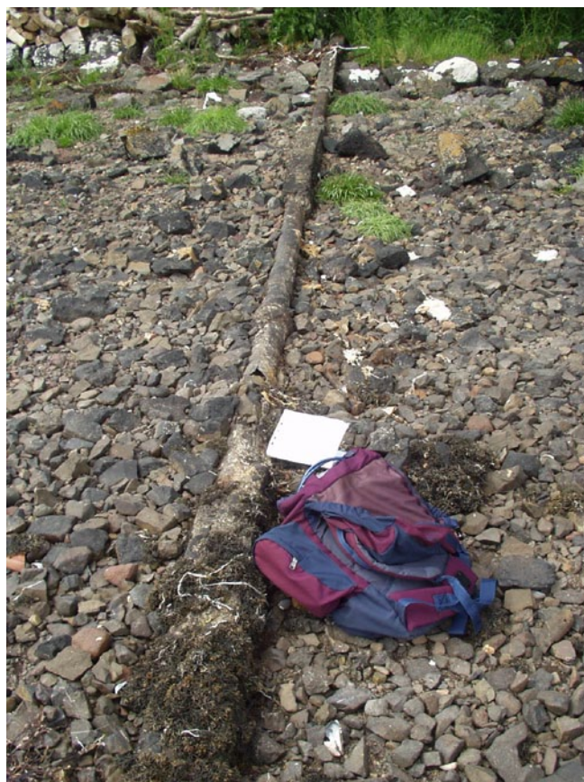
Figure 9. 10cm cast iron pipe
