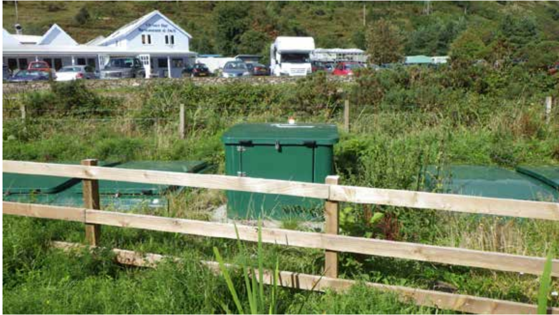
Fig 19. Septic tank at Loch Fyne Oyster Restaurant. Associated with waypoint 130.
