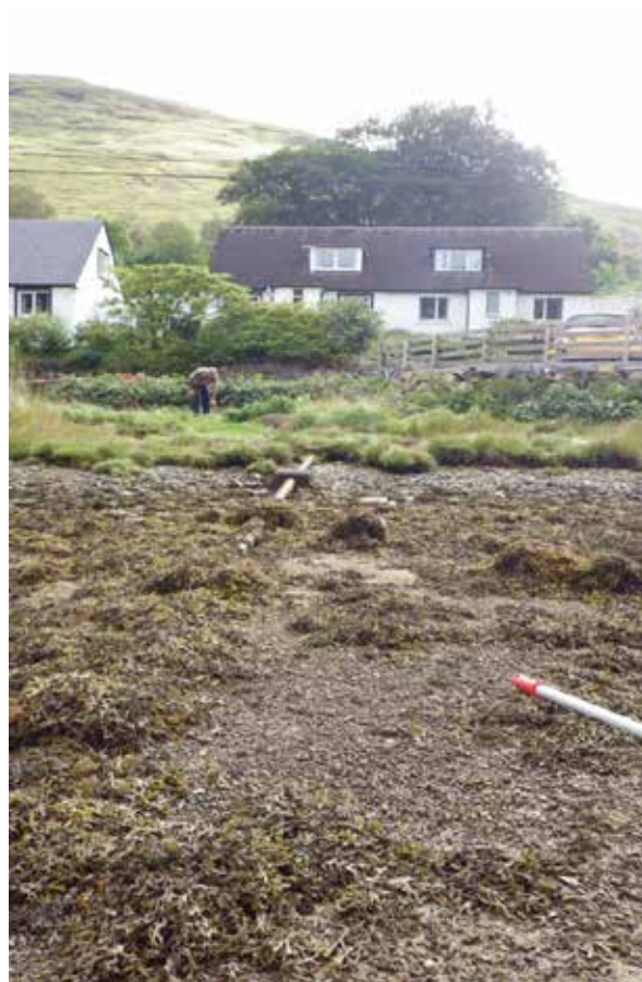
Figure 10. Metal pipe from houses, no discharge. Associated with waypoint 49.
