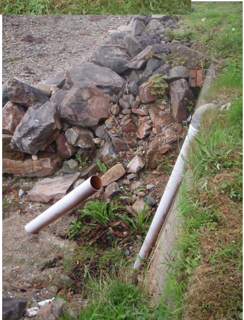
Figure 11. Discharge pipe for tank 2
