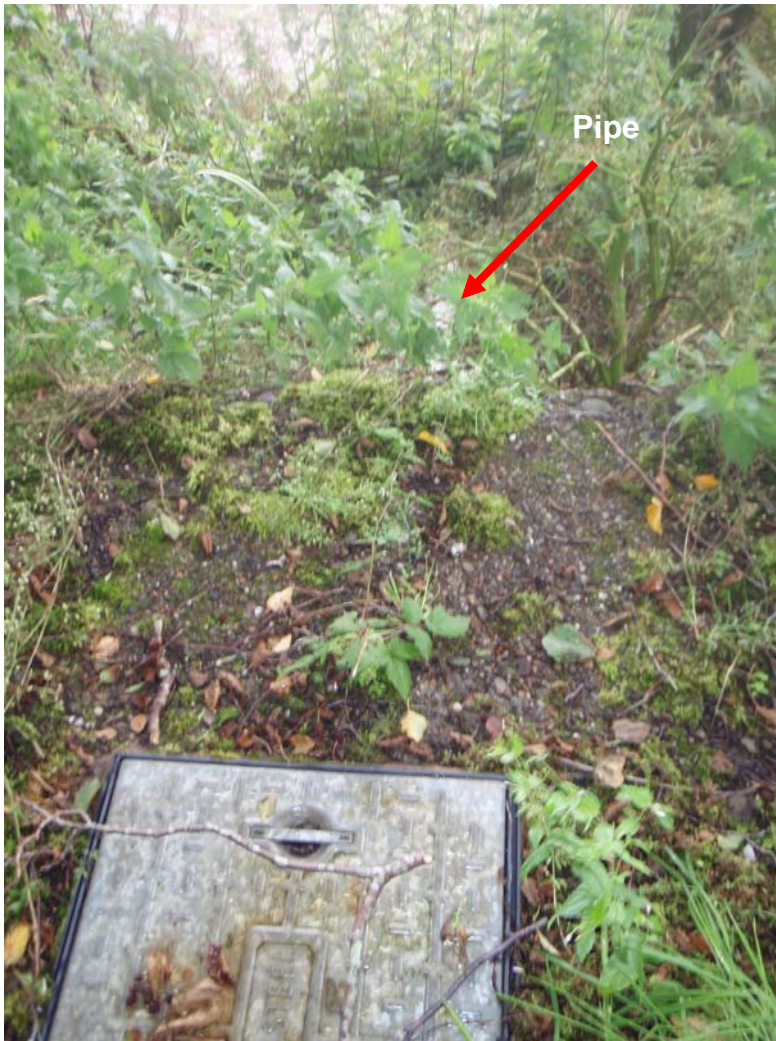
Figure 8. Septic tank with outlet pipe
