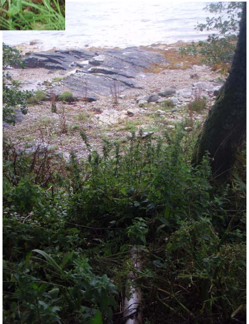
Figure 9. Discharge pipe for tank above
