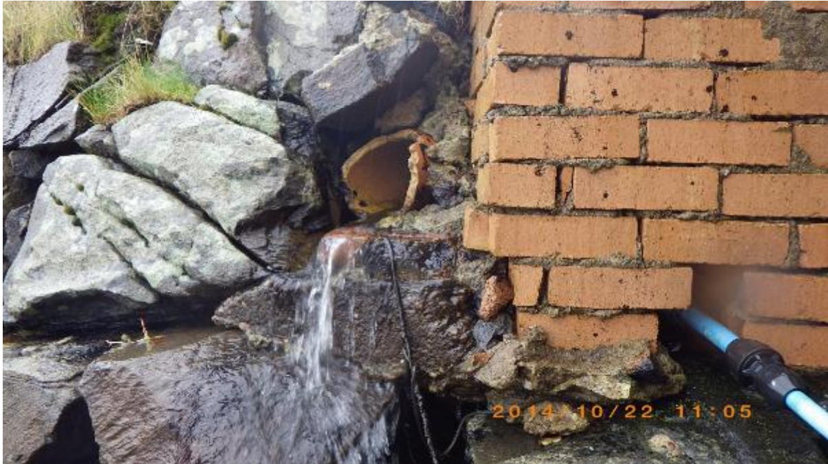
Figure 17. Associated with waypoints 84 and 85. Location of unplanned freshwater sample SFFW16 from broken pipe.
